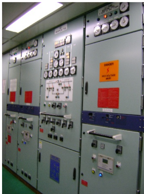
One of the main electric power distributors.
