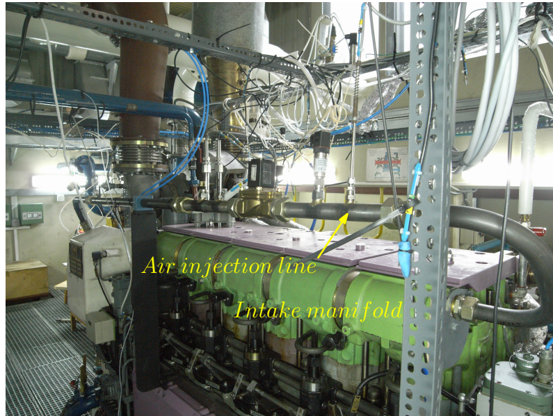
Figure 2.7: The air injection supply line as it enters the intake manifold at the right side
