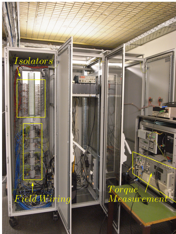
Figure 2.10: The cabinet in the Control room
