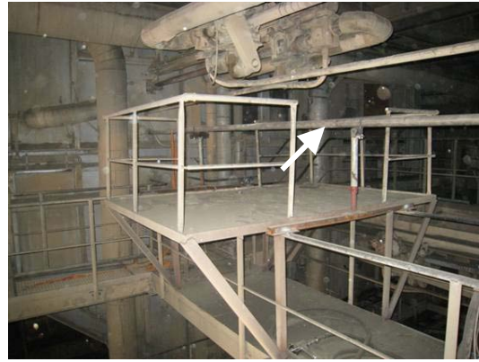
Fig. 6.4: View of the water-cooled pyrometer, level 26.5m
