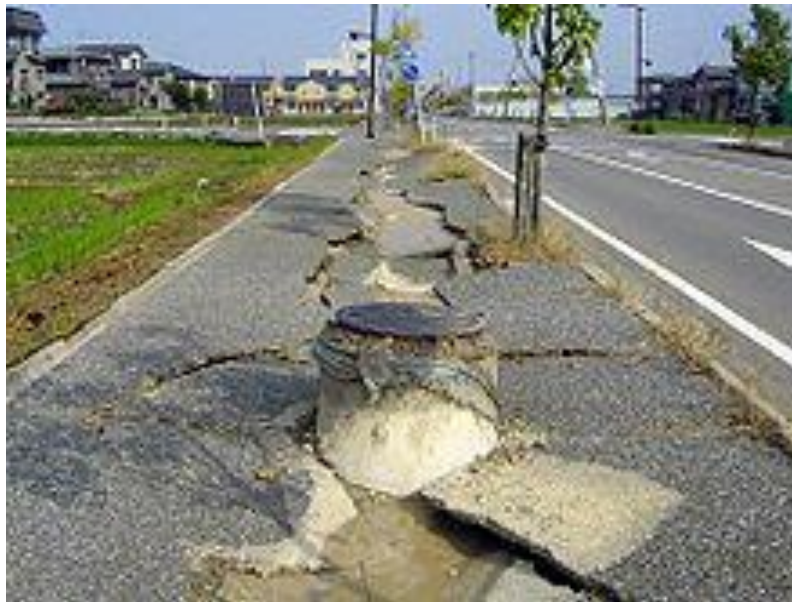
Figure 3.4.2: Effects of soil liquefaction after the 2004 Chūetsu earthquake
