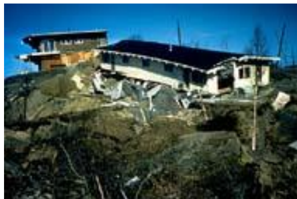
Figure 3.4.3: Displacement and tilting of houses due to soil liquefaction in the Turnagain Height area of Anchorage during the 1964 Alaska Earthquake
