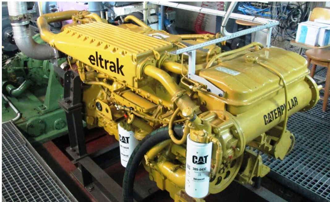
Figure 3.21: CAT marine diesel engine at LME
