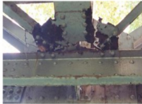
Figure : Bridge Corrosion
