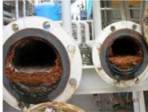
Figure : Pipe Corrosion and Fouling
