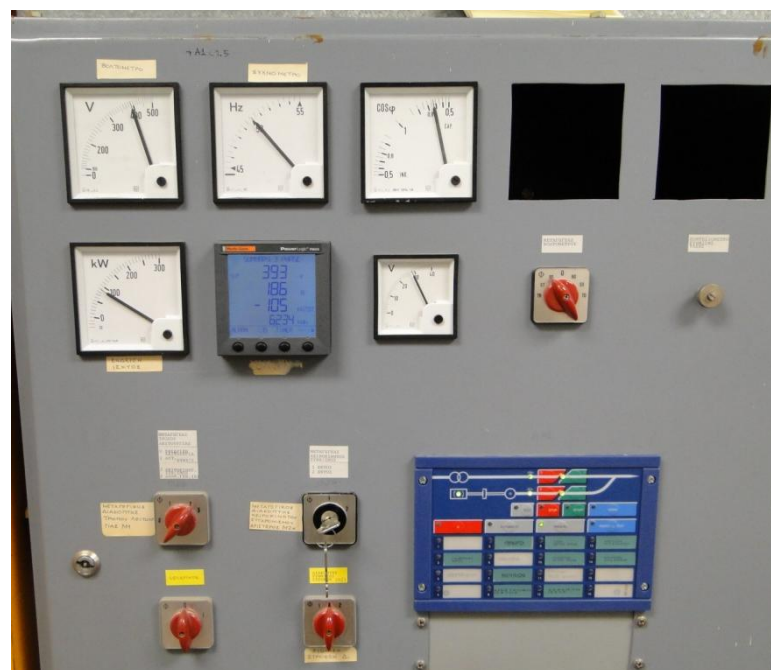
Figure 7.3.1. Front panel of electric generator's control unit
