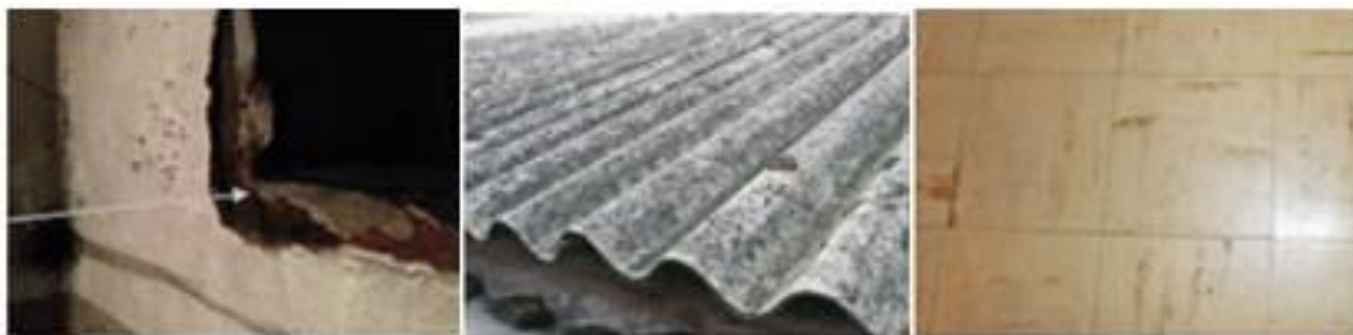
Figure 28 Amiante non friable : joints, fibro-ciment, colle
