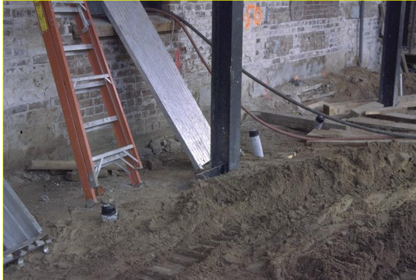
Figure 3.10: EQ-drains installed under an existing structure (Historic Charleston Courthouse, Geotechnics America, Inc.).
