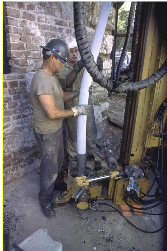
Figure 3.9: Restricted access drilling equipment and EQ-drain installation (Historic Charleston Courthouse, Geotechnics America Inc.).
