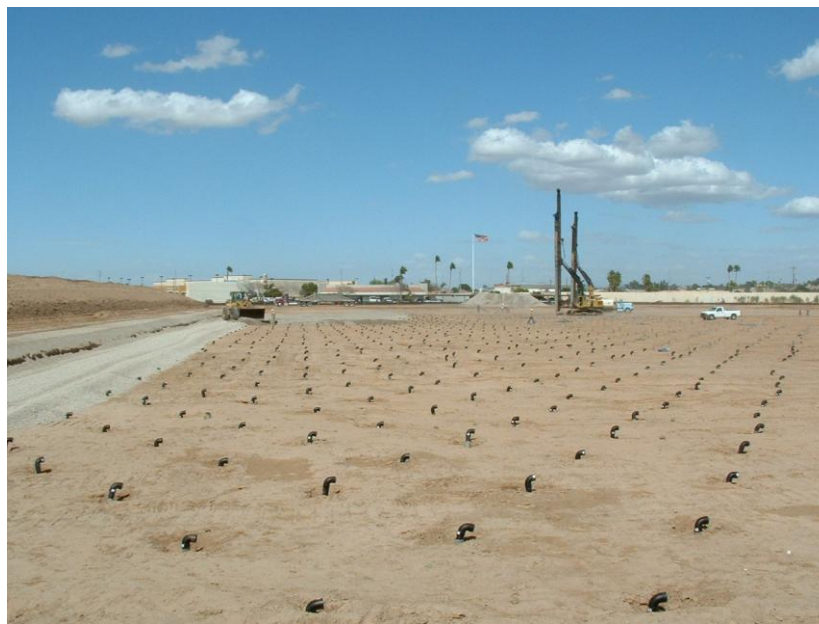
Figure 3.7: Finished EQ-drains with all elbows oriented in the same direction (Home Depot Yuma project, Nilex Corporation).
