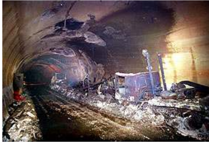
Figure 6-1 [Kum04]. Mont Blanc tunnel fire.
