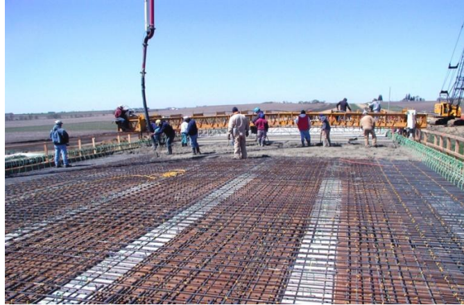
Fig.3. Iowa bridge deck USA; steel reinforcement of concrete slab nanoproccessed to develop anticorrosion properties and enhance mechanical capabilities, year 2011 [6]
