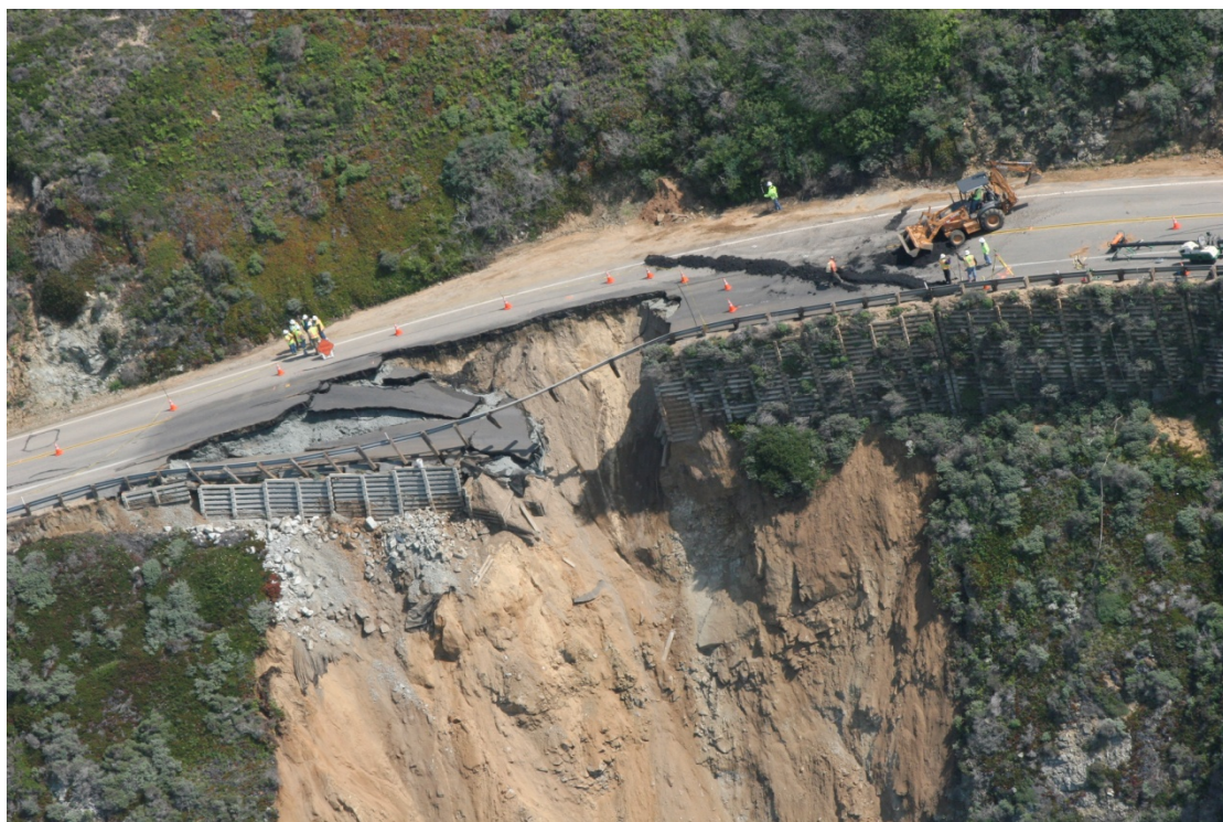
Figure 1.2: Slope instability effects on the infrastructure (California, 2011).
