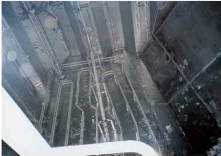
Figure 7.26 – Heating coils in chemical tanker
