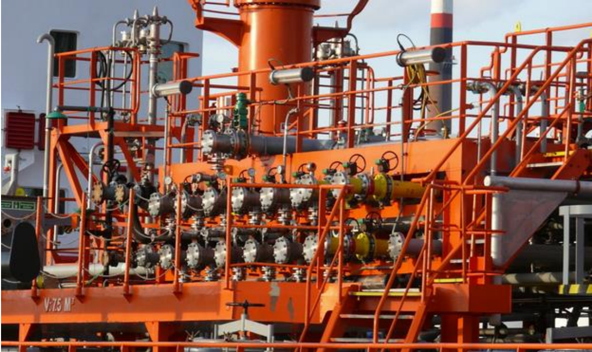
Figure 7.1 – Fully segregated ship manifolds
