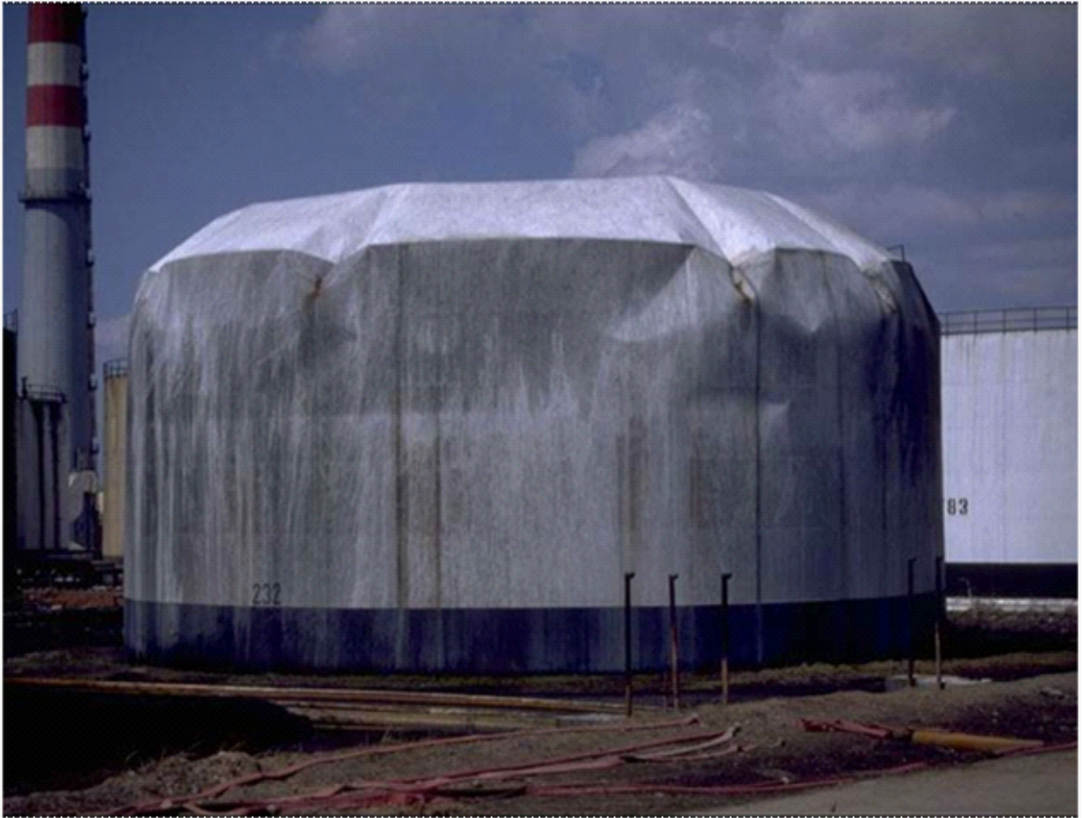
Figure 19: Roof damage by liquid sloshing (Hosseinzadeh (2008))
