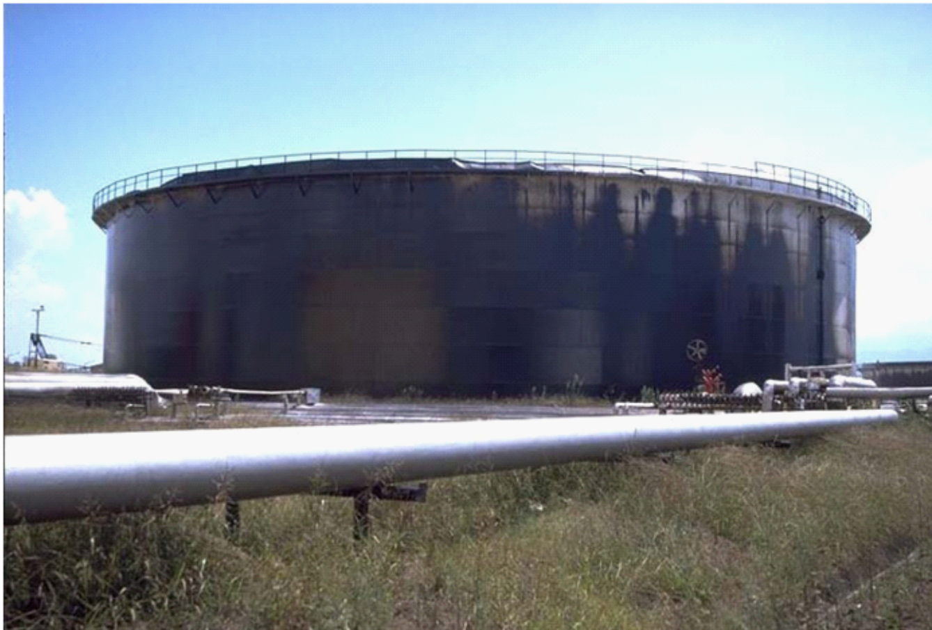
Figure 10: Overtopping of tank wall due to sloshing and failure of perimeter seals ( http://nisee.berkeley.edu/turkey/Fturkch4.pdf )
