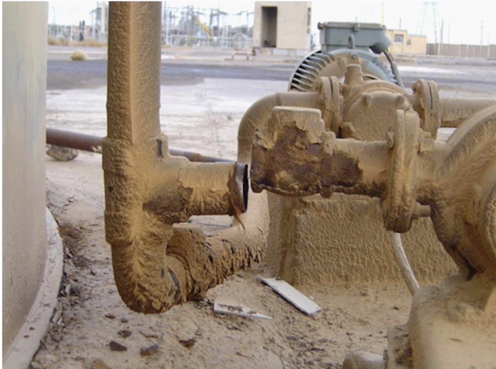
Figure 20: Failure of connections between piping and tank wall (Seyed-Razzaghi and Eshghi (2004))
