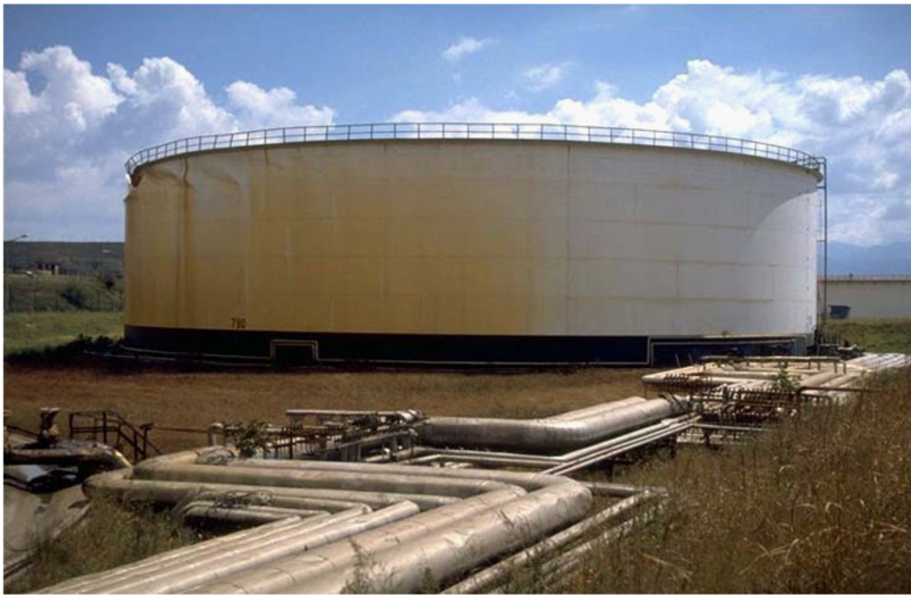
Figure 11: View of tank wall damage. ( http://nisee.berkeley.edu/turkey/Fturkch4.pdf )
