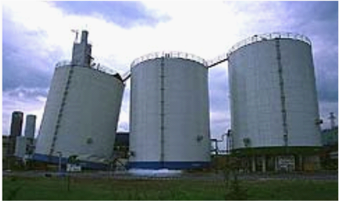
Figure 12: Liquid gas plants at the Habas plant ( http://nisee.berkeley.edu/turkey/Fturkch4.pdf )
