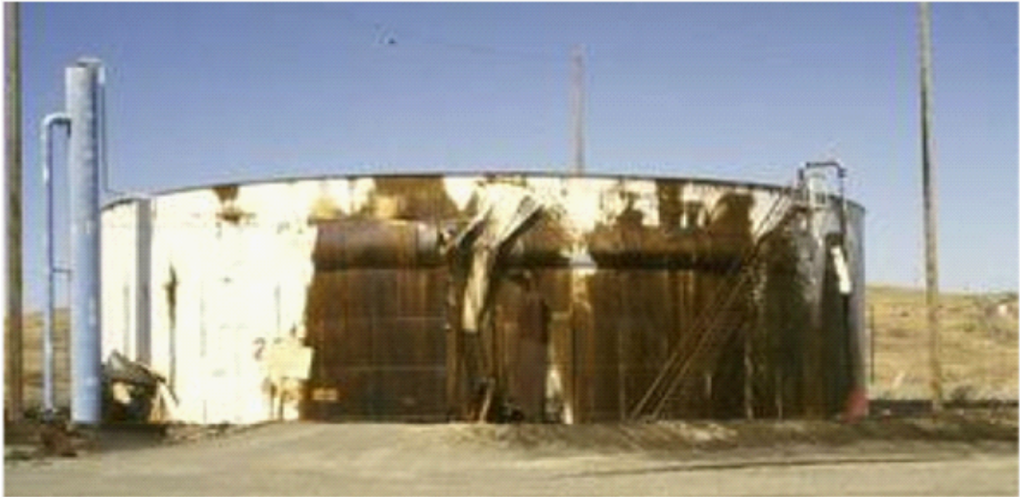
Figure 9: Damage to Shell Oil tanks, Chevron Coalinga Station #4, north of Coalinga ( http://nisee.berkeley.edu/elibrary/Image/S5813 , Karl V. Steinbrugge Collection: S5813)
