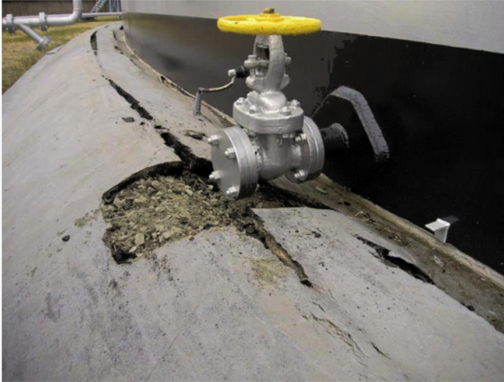
Figure 16: Tank settlement due to liquefaction around the foundation (Zama S et al. 2012)
