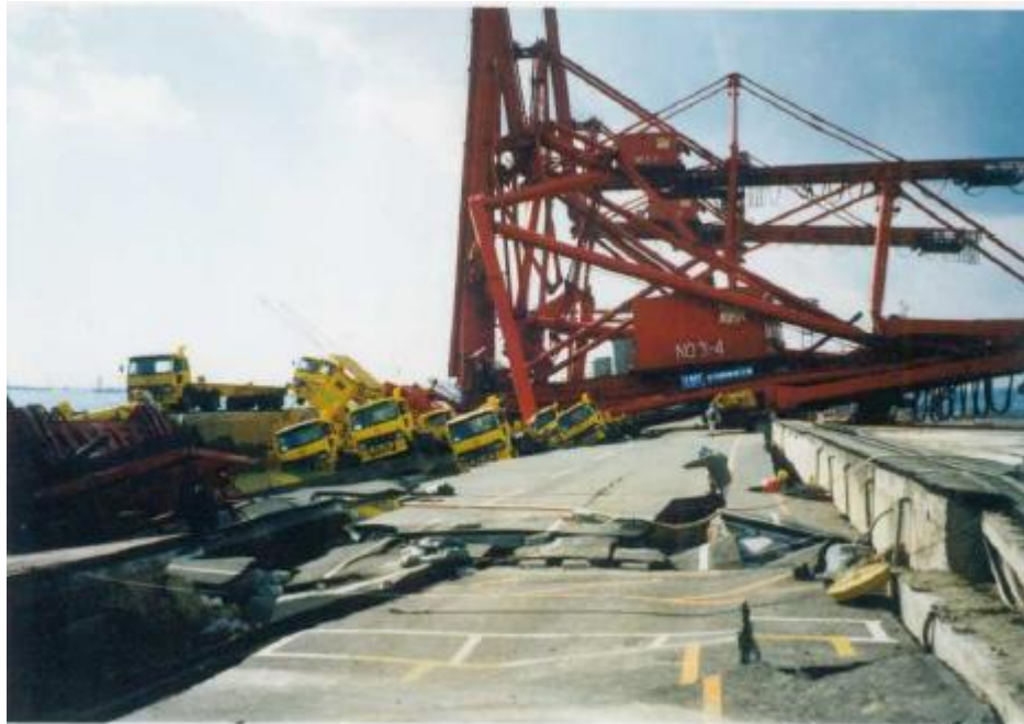
Figure 2.21: Damage to a quay wall at the Port of Kobe during the 1995 Hyogo-ken Nanbu Earthquake
