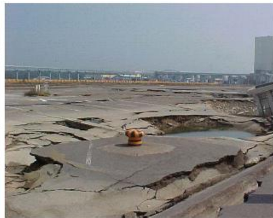
Figure 1.6 : Damages at the waterfront because of quay wall's displacement in 1999 Chi Chi earthquake
