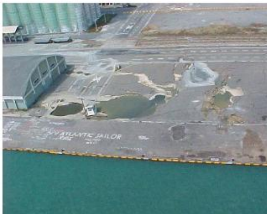
Figure 1.5 : Soil deformation behind quay wall at the port of Taichung during the 1999 Chi Chi earthquake
