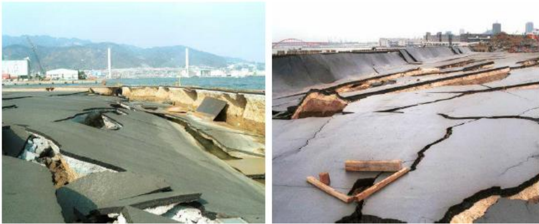
Figure 1.2 : Substantial damages in the pavement, placed in the foot of quay walls during Kobe, Japan 1995 earthquake
