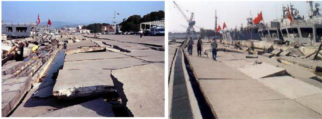
Figure 1.4 : Damaged quay walls at Navy Seals' base of Gölcük in the 1999 Kocaeli earthquake in Turkey
