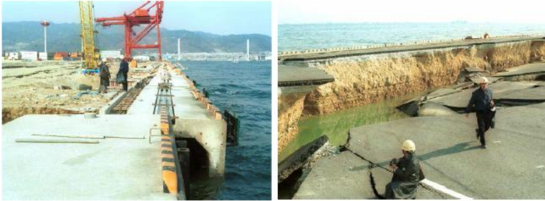
Figure 1.1 : Quay walls displacement and incline to the sea at Kobe, Japan 1995 earthquake
