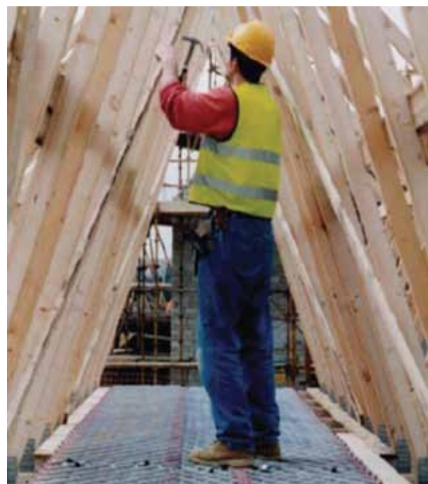
Safety decking system now complete providing a lightweight platform and an effective fall prevention system.
