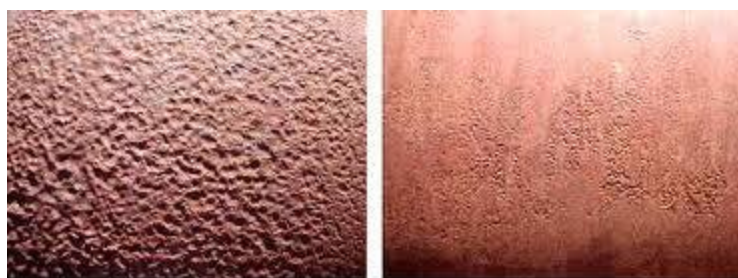
‘General Corrosion patterns’
