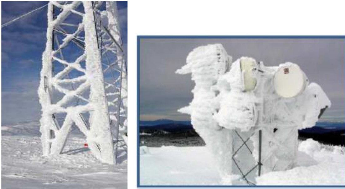
Figure 1.6: Failure of telecommunication towers
