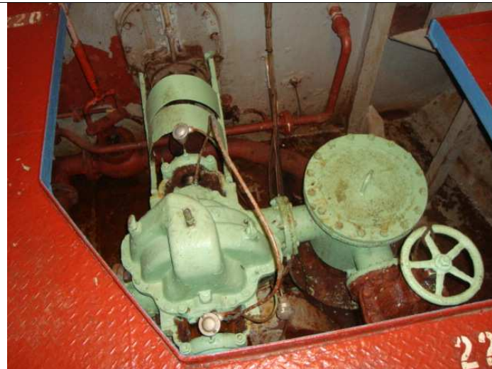
PUMP IN LOWER PART
