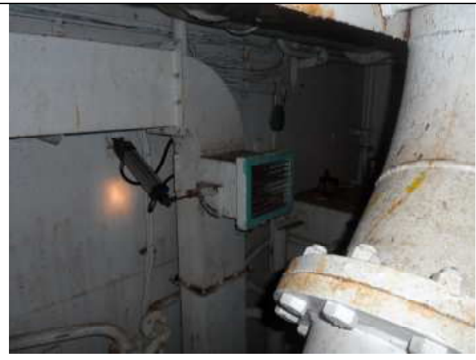
VENTILATION CONTROLLED REMOTELY
