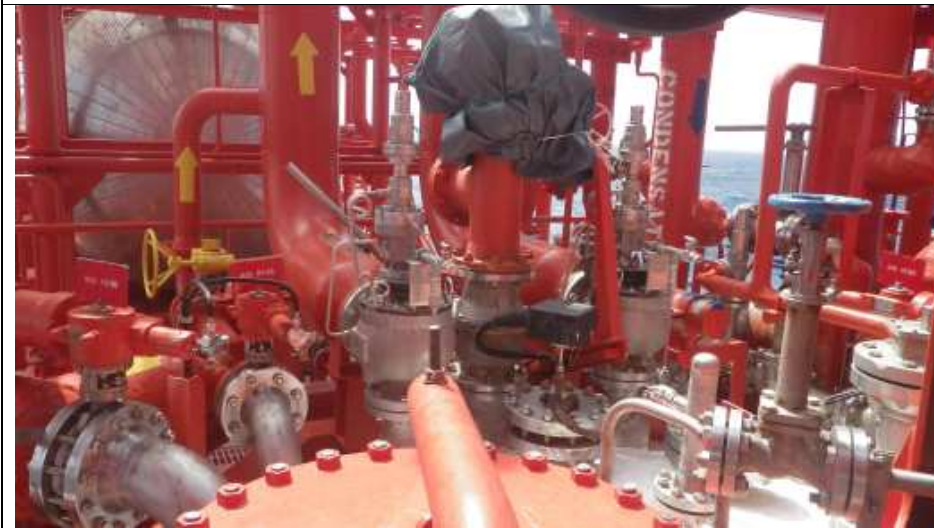
FITTINGS ON TOP OF THE CARGO TANK
