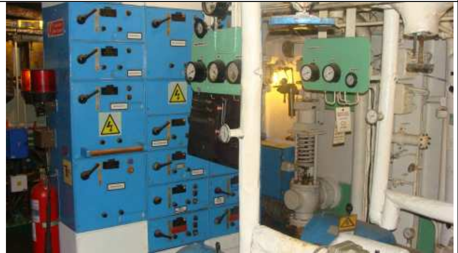
ADDITIONAL ELECTRICAL INSTALLATION
