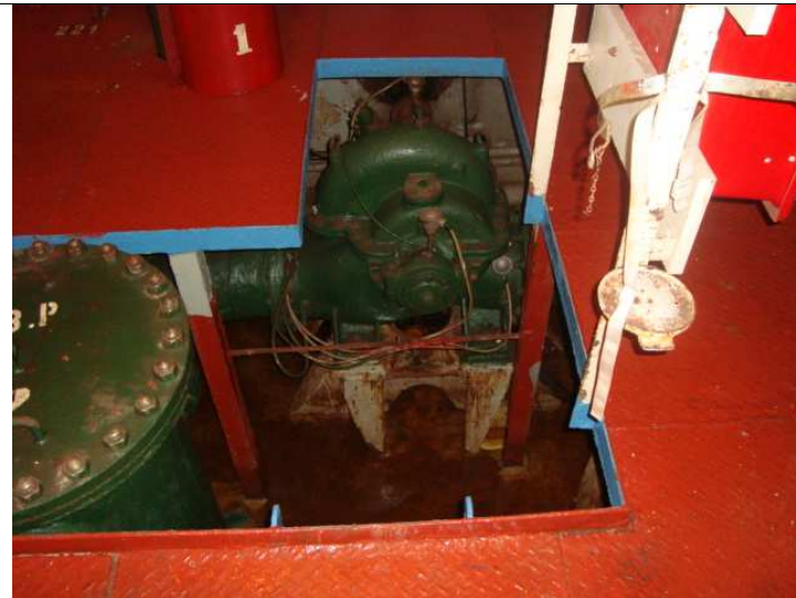
PUMP IN LOWER PART
