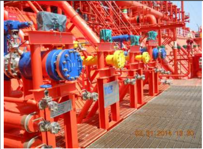
CARGO PIPING MANIFOLDS
