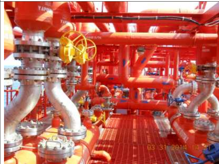
PIPING ON DECK
