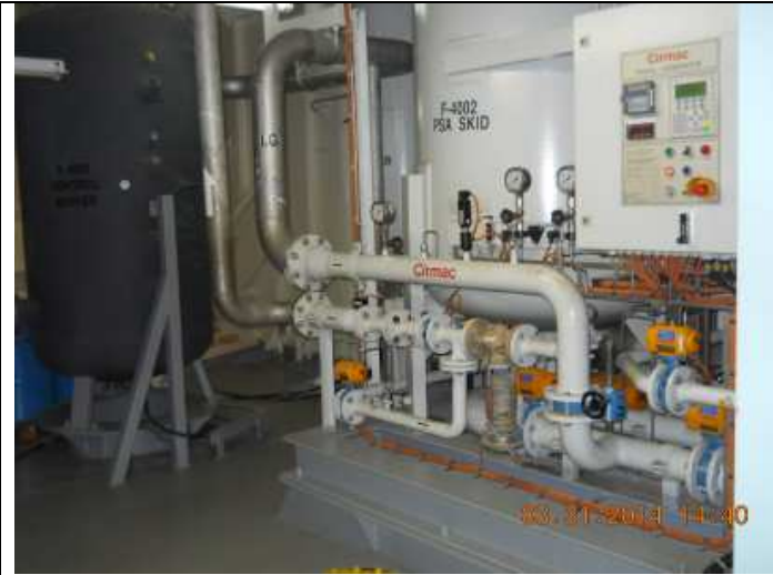
NITROGEN GAS GENERATOR
