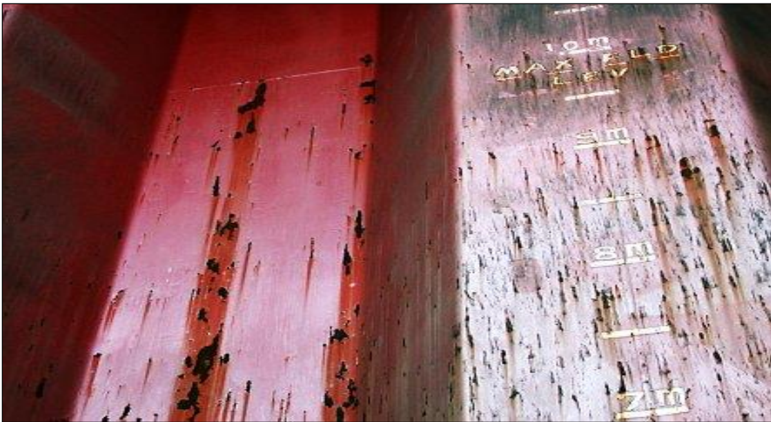
Figure 1.2: Pitting Corrosion on the sides of a Bulk Carrier's Cargo Hold [5]
