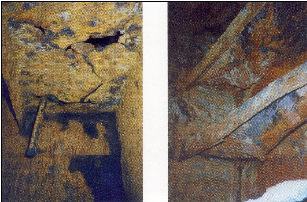
Figure 1.8: Corrosion of longitudinal stiffeners in ballast tanks (fully unprotected) found near the transverse web region [1]
