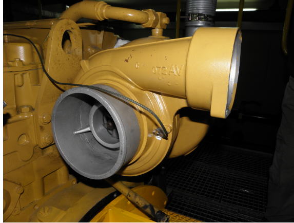
Figure 2-14: Turbocharger speed measuring sensor as installed on the DE of the HIPPO-1 testbed.
