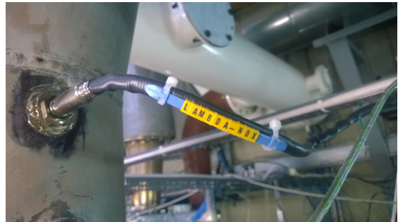
Figure 2-11: The SmartNOx sensor as installed at HIPPO-1 testbed
