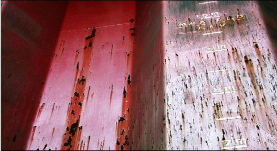
Figure 1.2.: Pitting Corrosion on the sides of a Bulk Carrier 's Cargo Hold [5]
