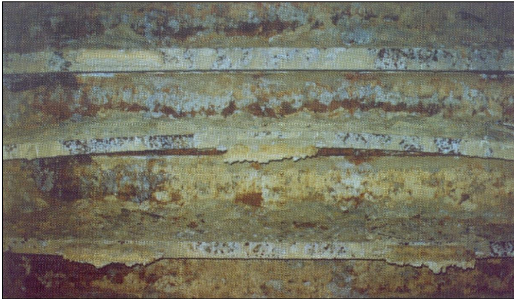
Figure 1.7: Corrosion of longitudinal stiffeners in ballast tanks (fully unprotected) [1]
