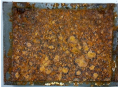
The corroded surface
