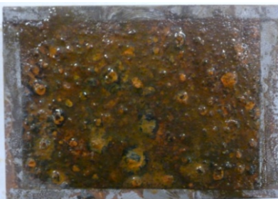
The corroded surface
