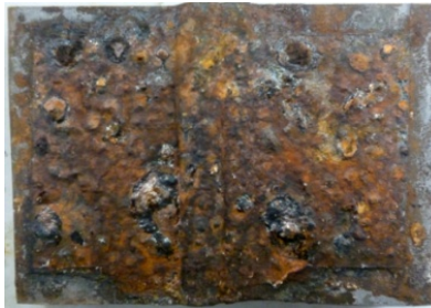
The corroded surface
