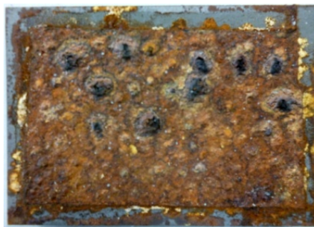
The corroded surface
