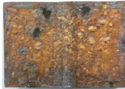
The corroded surface
