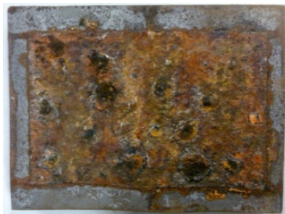
The corroded surface
