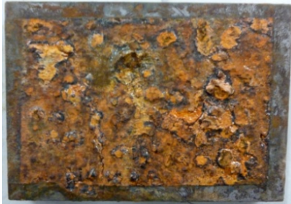
The corroded surface
