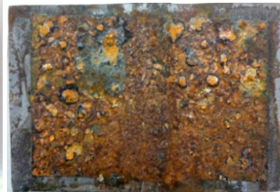
The corroded surface
