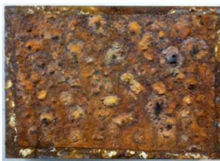
The corroded surface
