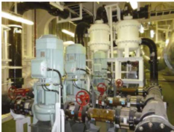
Figure 11: Wash water treatment system with GRE piping
