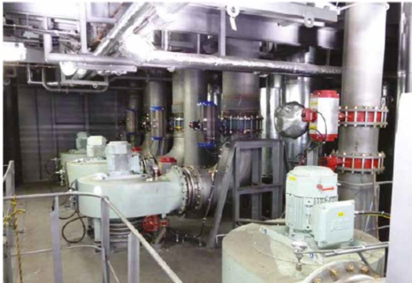
Figure 18: ID fans in exhaust ducts (Source courtesy of Hamworthy-Krystallon)
