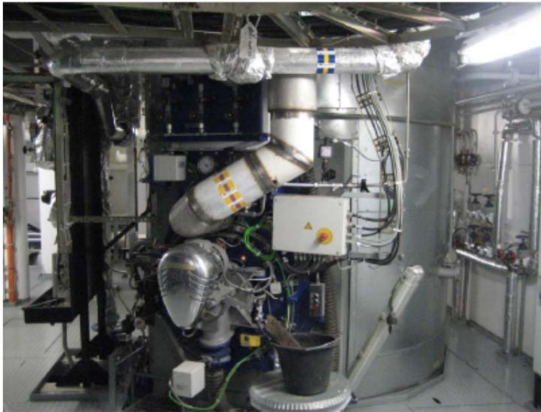
Figure 32: Image of the boiler
