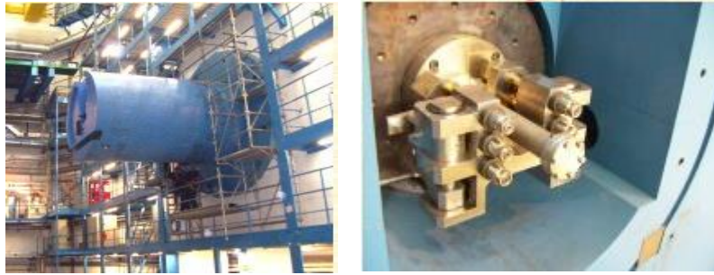
Figure 6.13: Left: The monobloc after installation. Right: Front view of the TAS collimator and the remotely controlled beampipe flange. [63]
