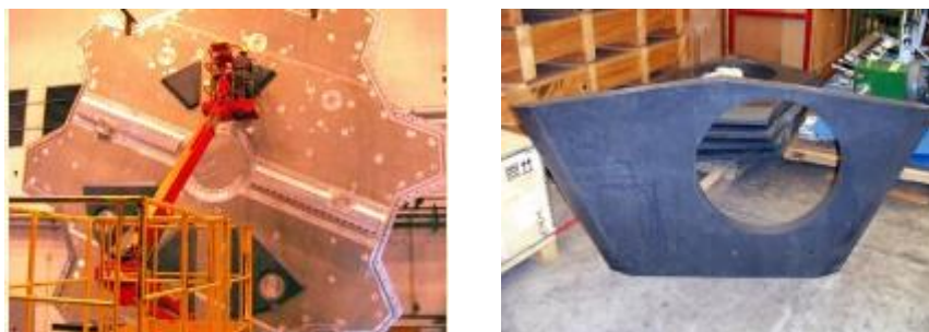
Figure 6.8: Left: Installation of JTV petals on the endcap toroid endplate. Right: A JTV petal segment in the front wall. [63]
