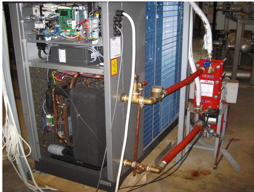
Figure 33 – Side view of the installed commercial heat pump before its retrofitting with the expander prototype.
