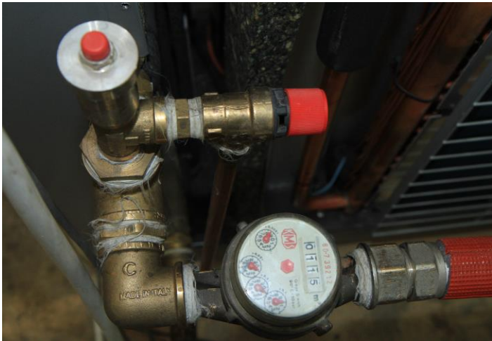
Figure 47 – Supply water flow-meter.
