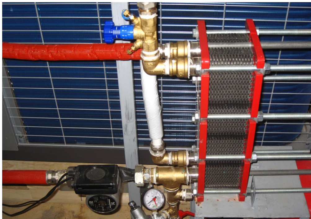
Figure 35 – Detail of the installed closed circuit supply water system – the plate heat exchanger, the circulation pump (black) and the manual adjustment valve (in blue) can be seen.
