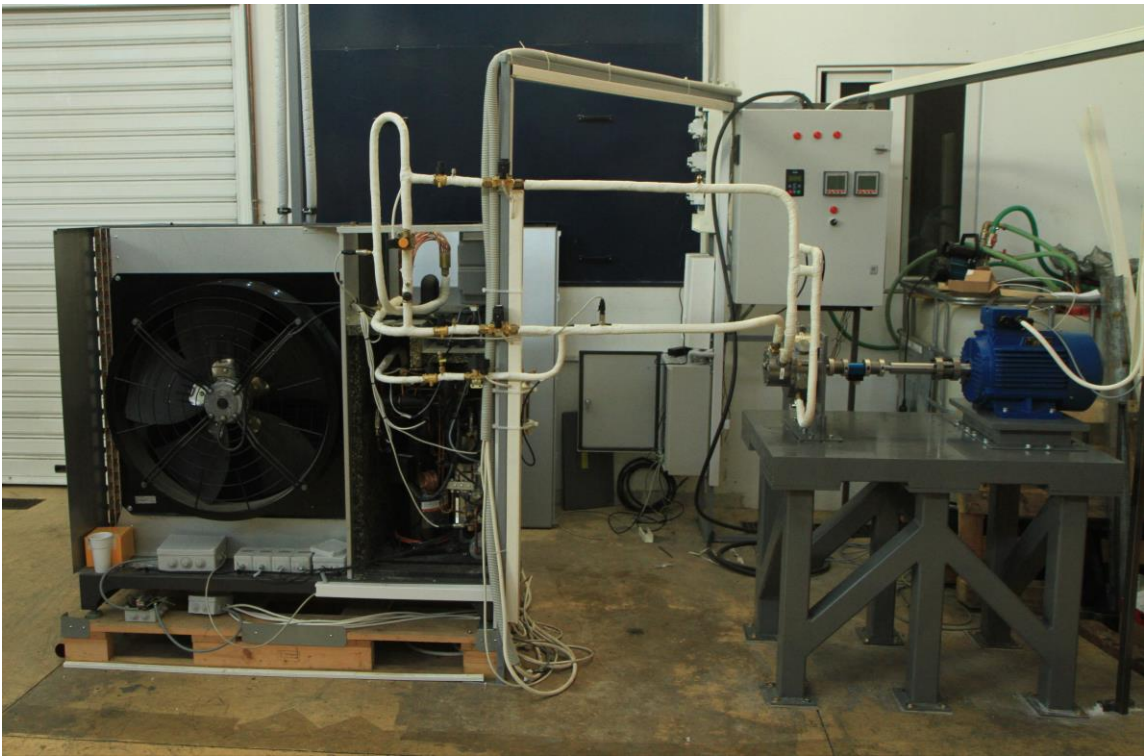
Figure 38 – The installed heat pump unit retrofitted with the expander prototype.
