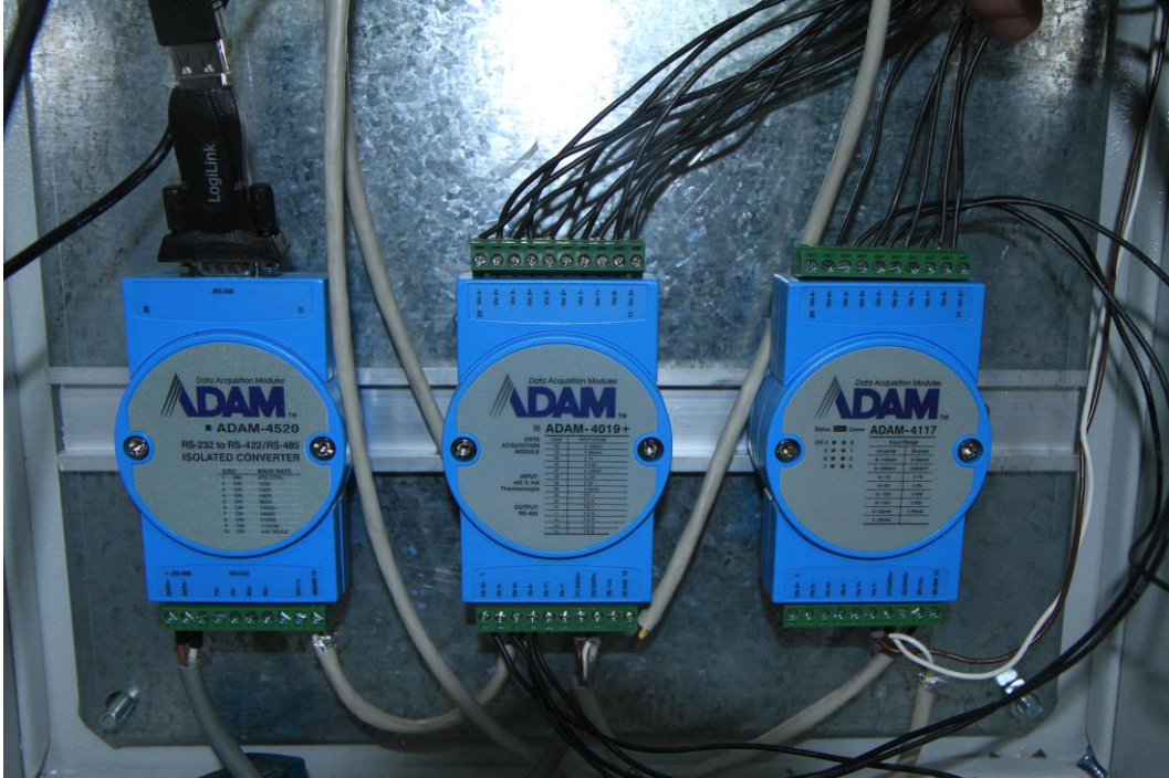
Figure 46 – ADAM data acquisition and control modules.
