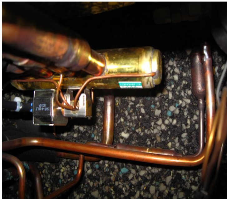
Figure 37 – Detail of the installed heat pump before its retrofitting with the expander The four-way valve QN2.
