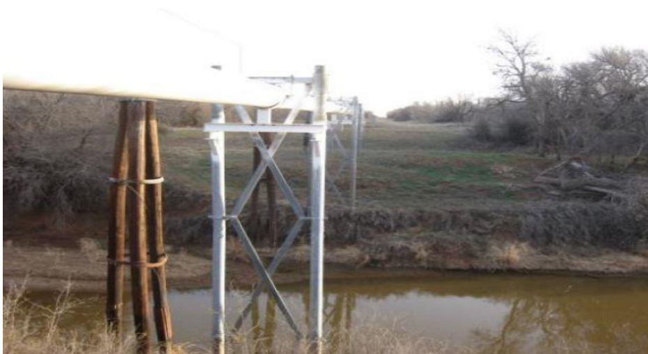
Figure 2.5: Pipeline support exposed to a soil liquefaction (Barry, Plains Mid American, 2014)
