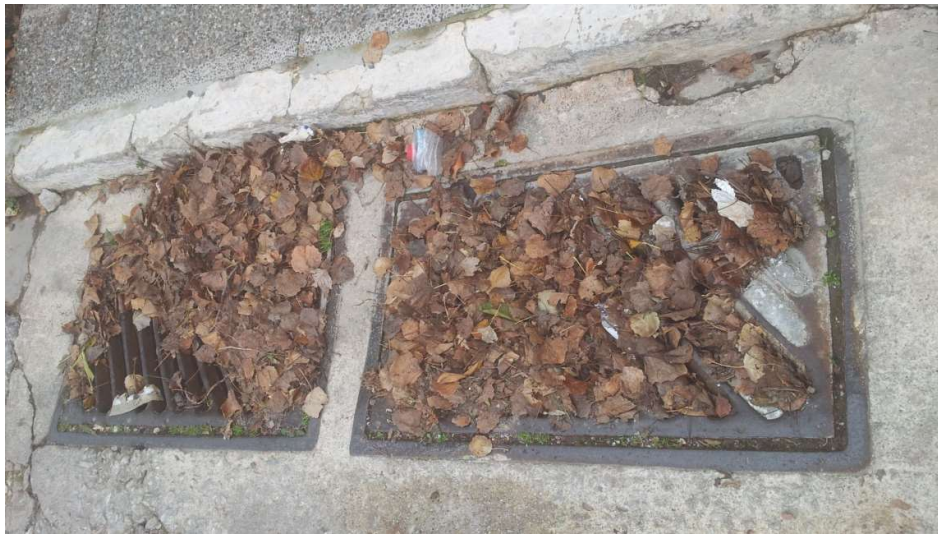
Figure 2.5. Clogging of sewer systems from tree leaves and litter (personal archive).
