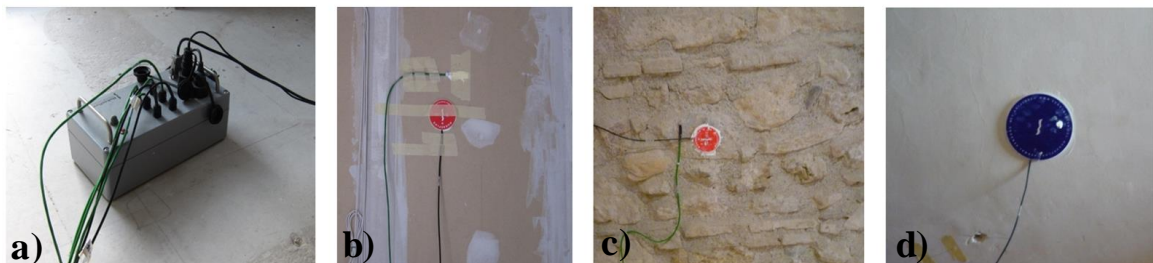
Figure 4.2 – Instrumentation: a) The TRSYS01 equipment and b) the temperature and heat flux sensor at the Wall A, c) the temperature and heat flux sensor at the Wall B and d) heat flux sensor at the Wall C.
