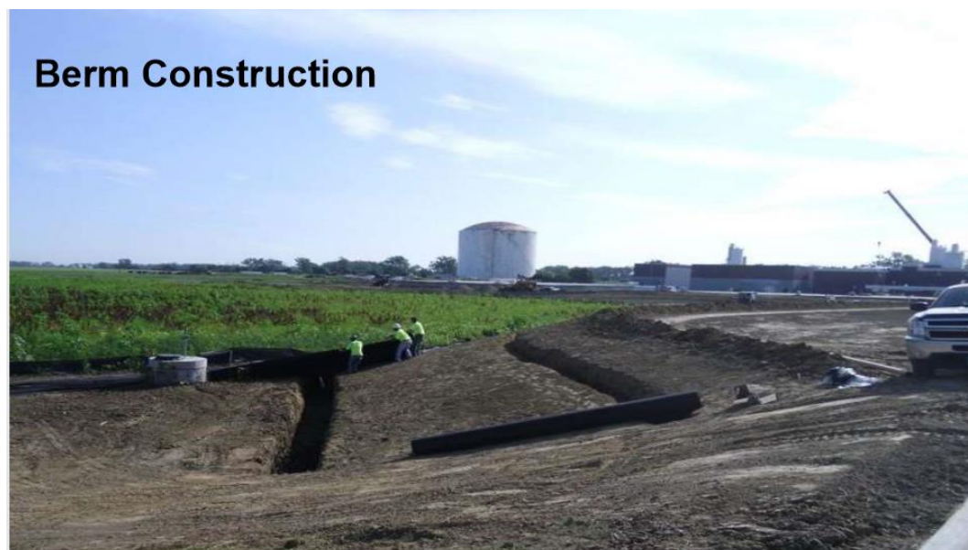
Εικόνα 3-5. Κατασκευή αναχώματος (Protection of Water and Wastewater Treatment Plants with FEMA Funding Assistance(2016), Session D4, Chris Koenig, Senior Project Manager)
