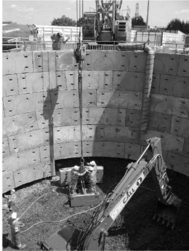
Figure.6 Erection of pre-cast segments for Ref. National Grid (2015). The ground is exposed prior to erecting the shaft lining (Faustin et al., 2013).
