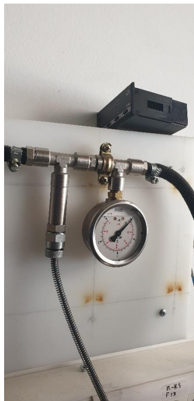
Figure 155 - Pressure and Temperature Gauge
