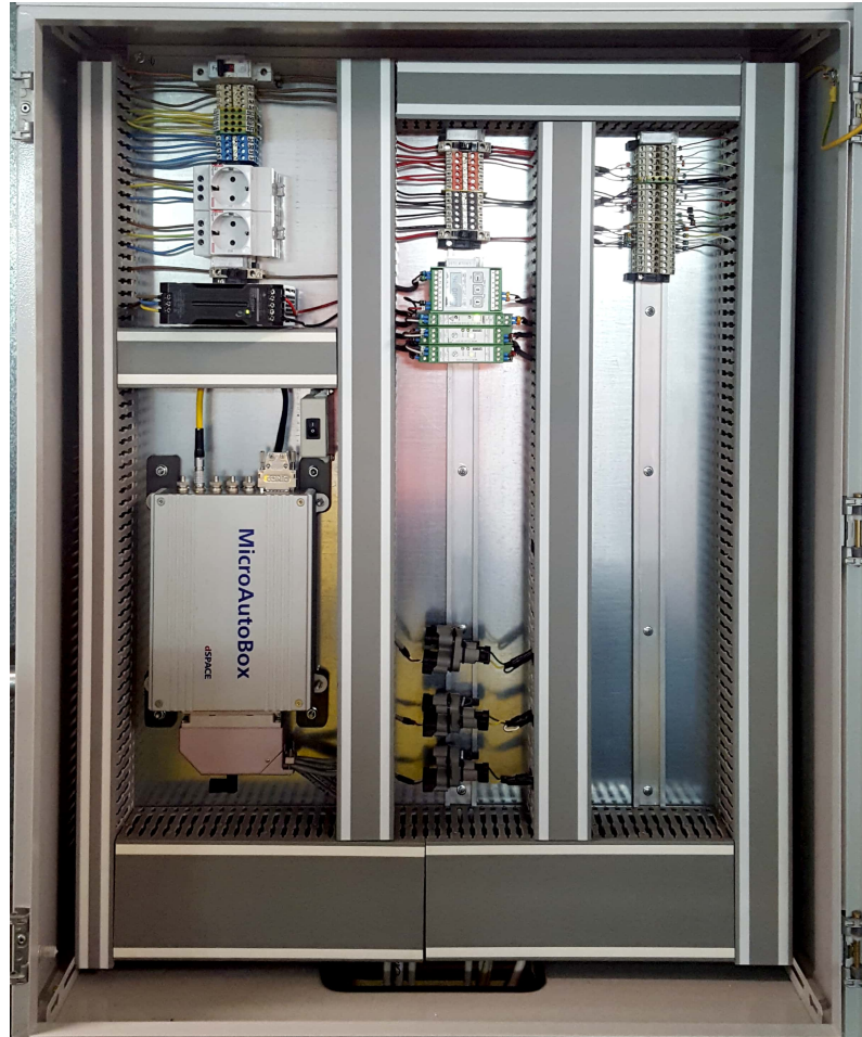
Figure 3.14: +Y12-H15 Electric Panel.
