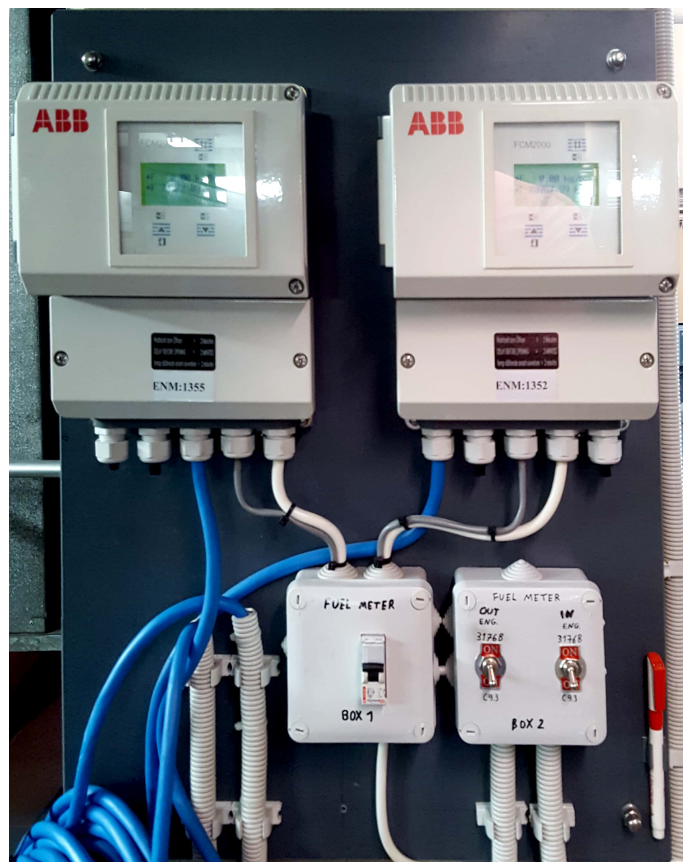
Figure 3.8: ABB Coriolis panel.
