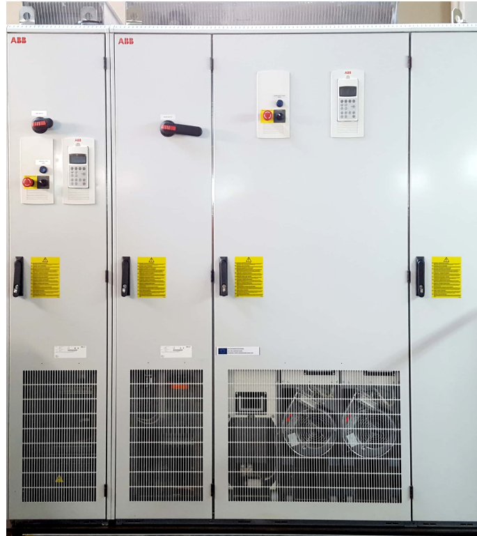
Figure 3.10: ABB ACS 800 controlling panels.
