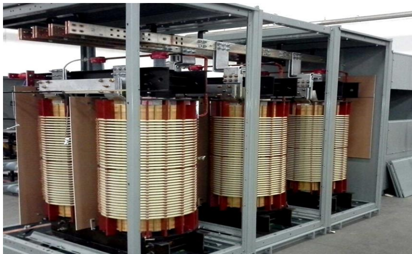
Figure 2.8 – Substation's Dry-type voltage transformers
