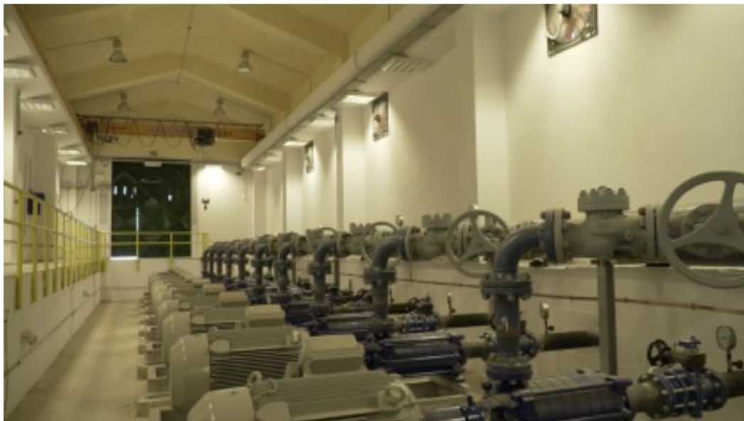
FIGURE 29: PUMPING STATION'S INTERIOR
