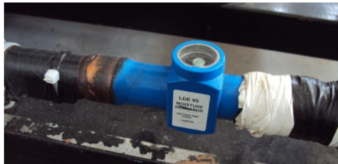
Figure 3.4: Installed sight-glass right before the pump suction port.
