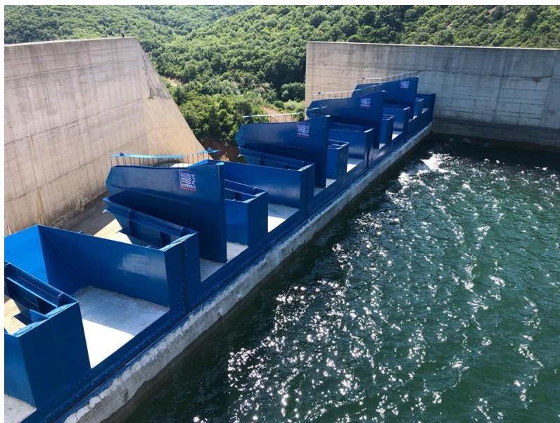
Figure 1: Combination of Piano Key weirs and Fusegates installed in Aisymi's Reservoir in Evros, Greece. (Source: https://www.evros24.gr/ )
