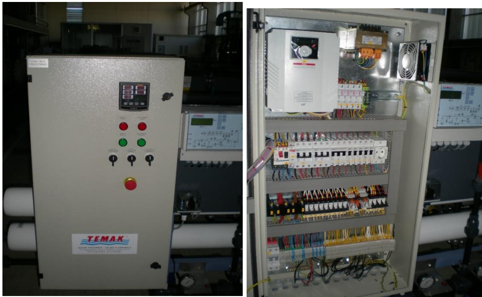
Figure 3.54 The switch board of the RO sub- unit (outside and inside view)
