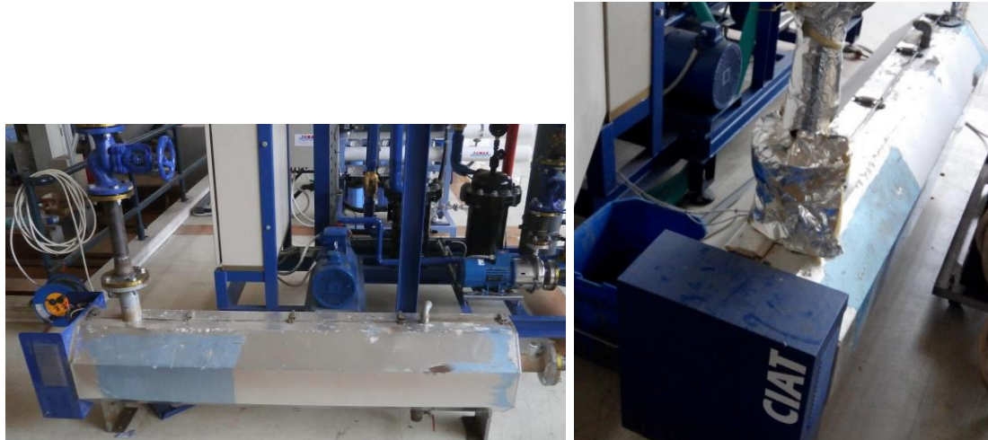
Figure 3.3 The electric heater of the heat cycle
