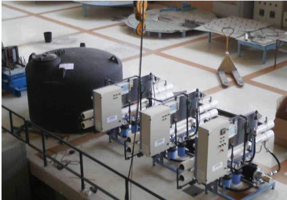
Figure 3.62 The installed RO unit system in the NTUA Laboratory of Hydraulic Turbomachines
