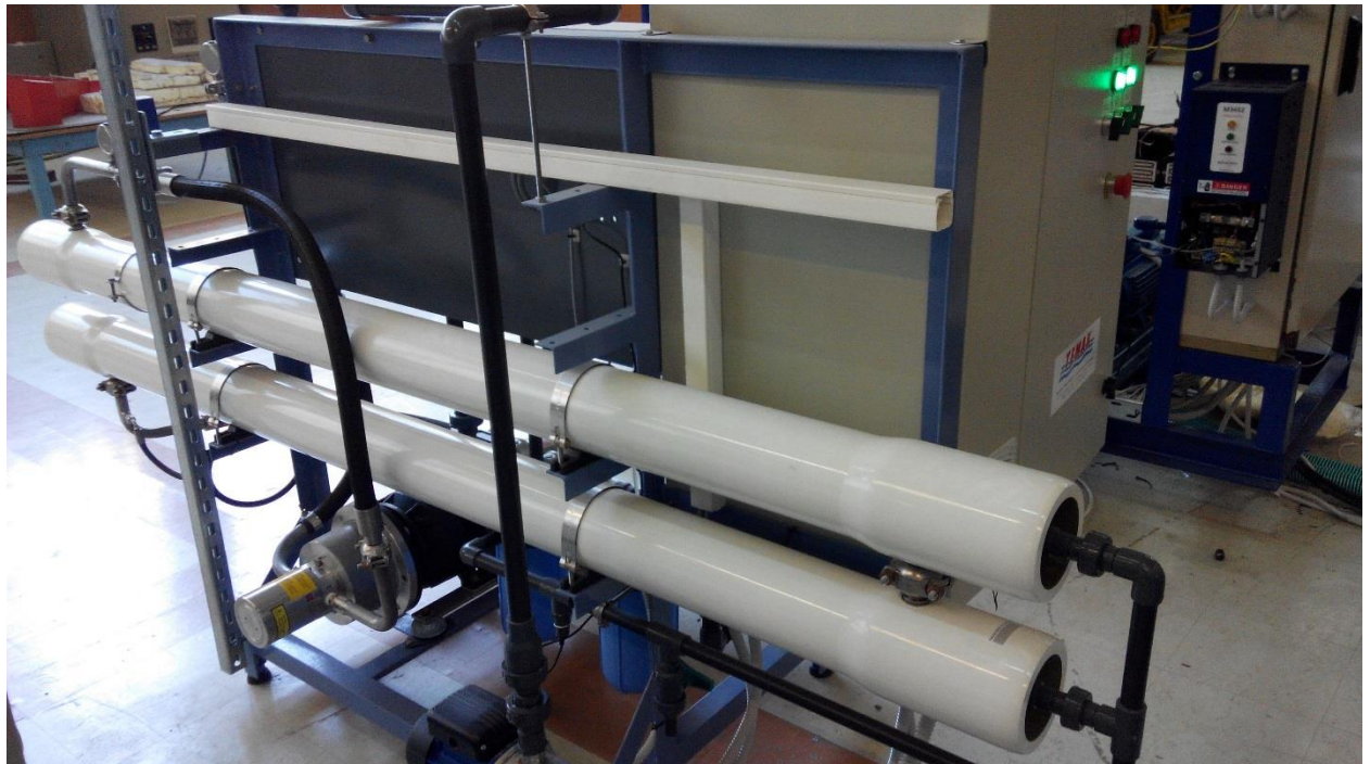
Figure 3.52 the sub- unit membrane vessels (membranes manufacturer Filmtec DOW company)
