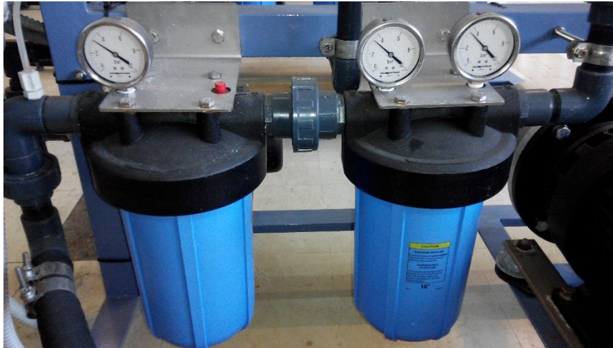
Figure 3.47 Filter housings on the sub- unit
