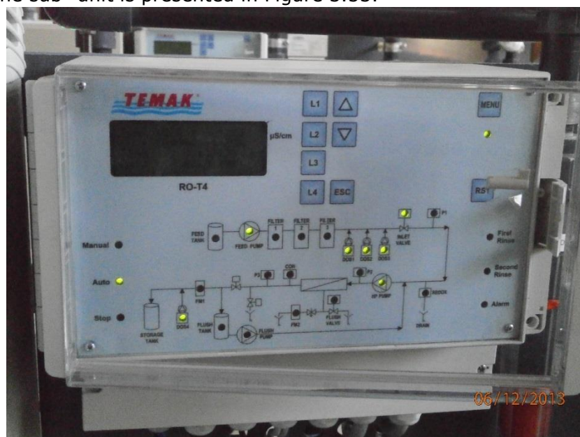
Figure 3.53 The sub- unit RO-T4 control panel (TEMAK company)
