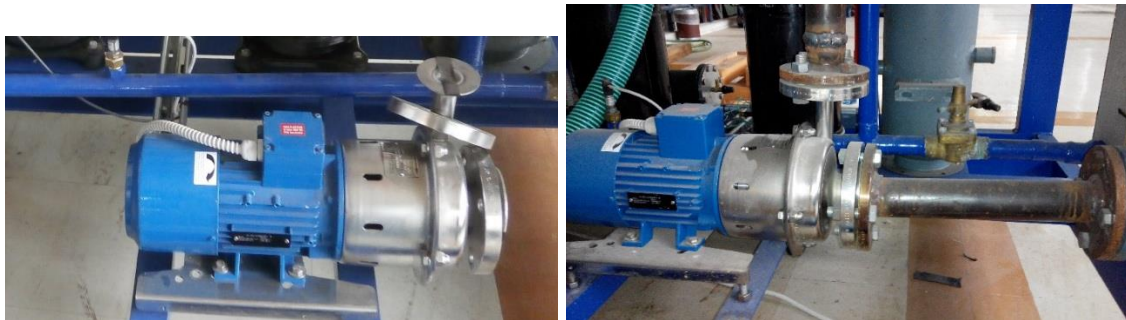
Figure 3.4 Centrifugal circulation pump of the heat cycle, Packo company, ICP2
