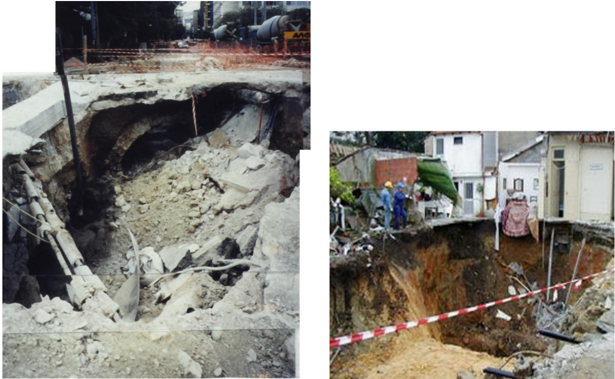
Figure 9: Photos of “chimney” failures and the resulting craters (“Athens Metro”, left; “Metro do Porto”, right; P. Marinos Lecture, 2014)
