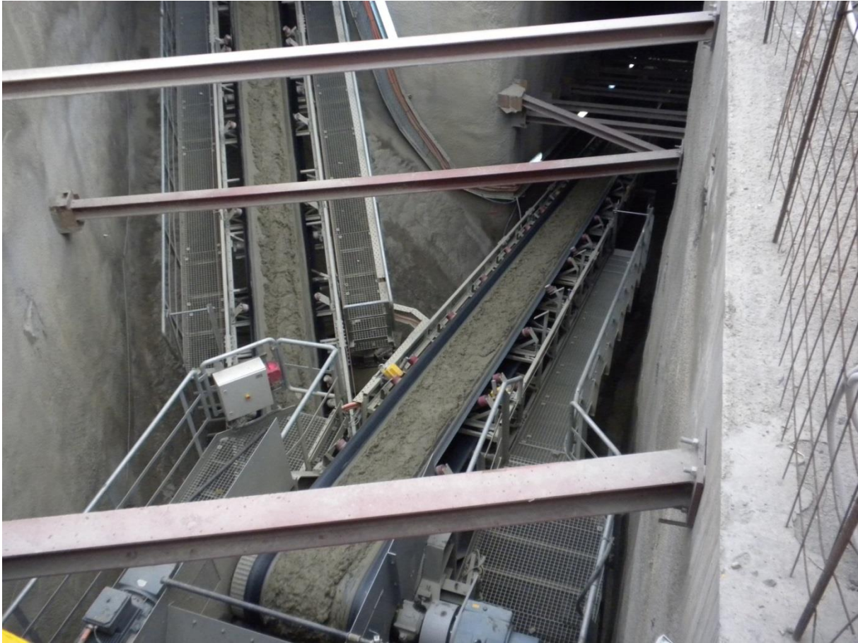
Figure 70: Field observation of EPB's conveyor belt of Athens Metro Line 3 Extension Project at Ag. Varvara Station (1).
