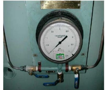
Scavenging air and exhaust receiver pressures.
