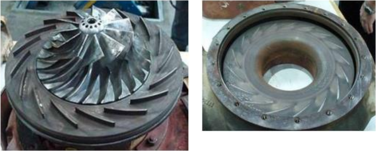
Figure 9: Compressor stage with typical fouling [1]
