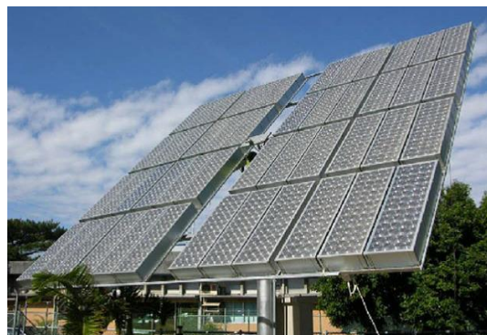
5 kW HCPV system (1st generation) at INER
