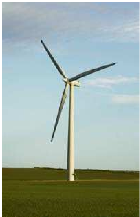
A horizontal axis wind turbine
