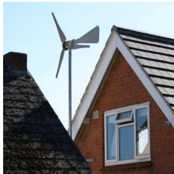
Residential wind power installation
