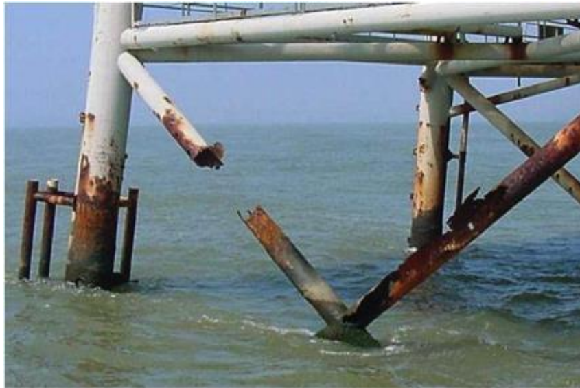
Figure 2.2: Corrosion of an offshore tower support structure
