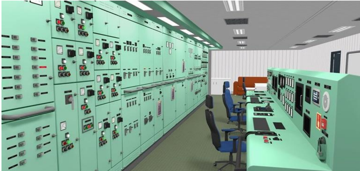
Fig. 1 Engine Control Room ( https://www.wingd.com )
