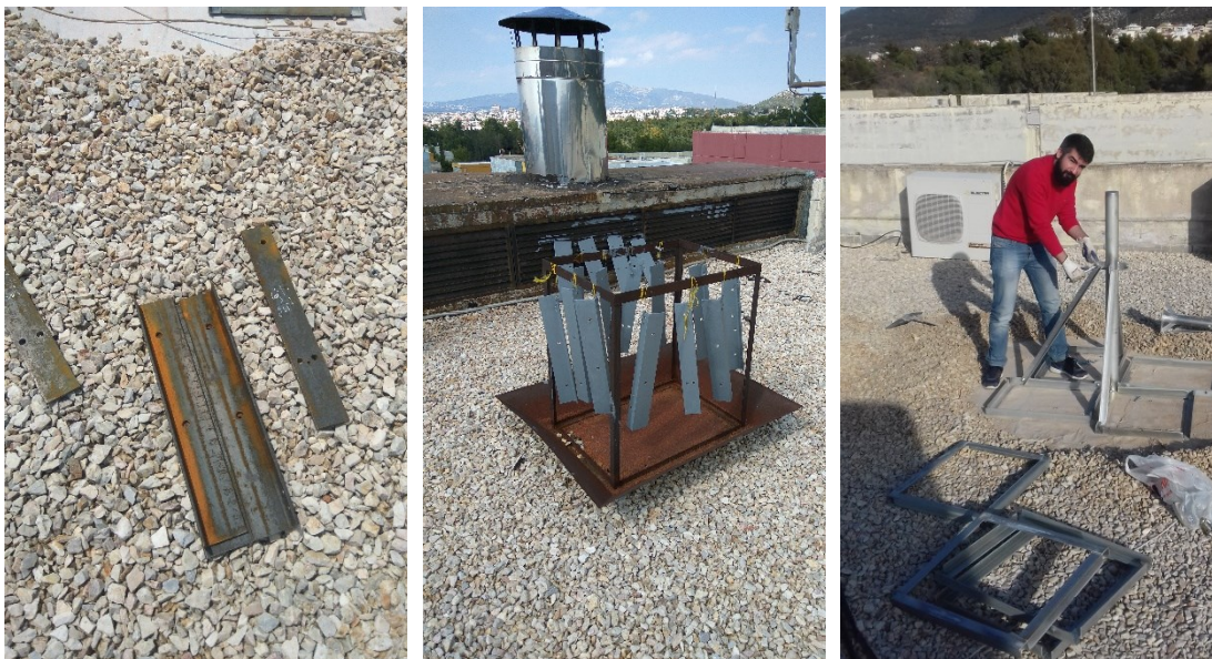
Figure 4-22: The construction of fully custom antenna mounts with integrated tracking functionality for Q-band
