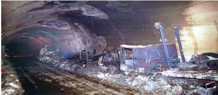
Figure 1.1 Structural damage of Mont Blank Catastrophic Tunnel Fire
