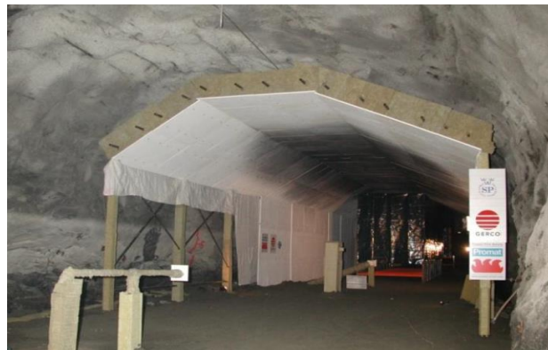
Figure 3.2. Applying fire protection in Runehammar Tunnel Fire Test, during fire tests of several MWs, (Ingason et al., 2011).
