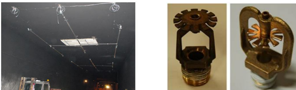
Figure 3.5. Deluge fire suppression system with standard spray and directional 180° nozzle, used in San Pedro Tunnel Experiment, Spain (Cheong et al., 2014).
