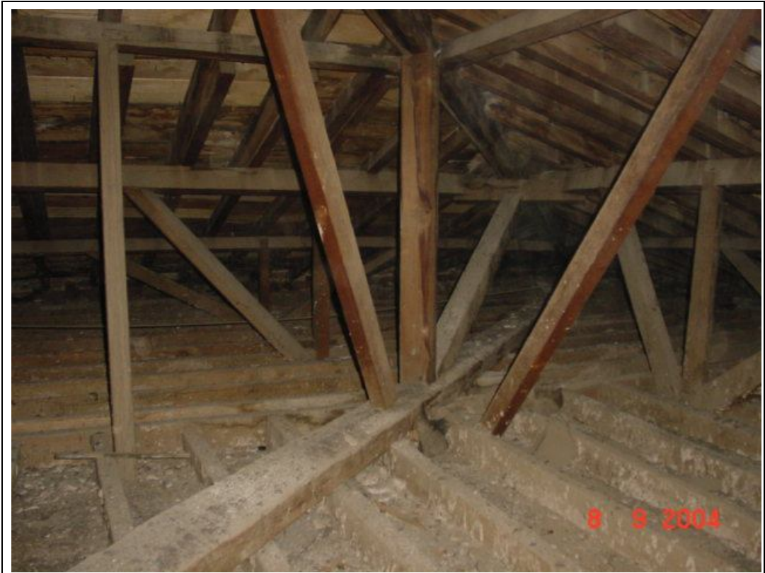
Description: Ph.46 – Part view of the main diagonal timber roof truss and the secondary trusses for the support of roof elements.
