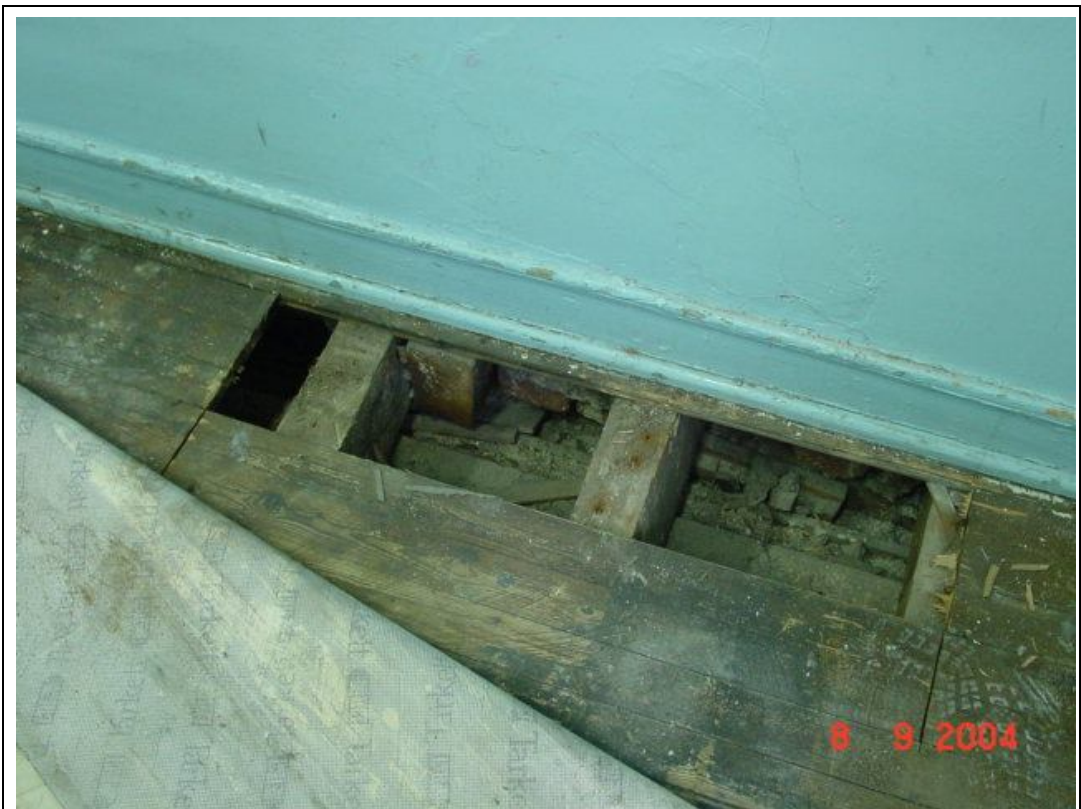
Description: Ph.55- Timber floor section at room O7 with the transverse timber beams being supported on the wall between rooms O7 – O8.
