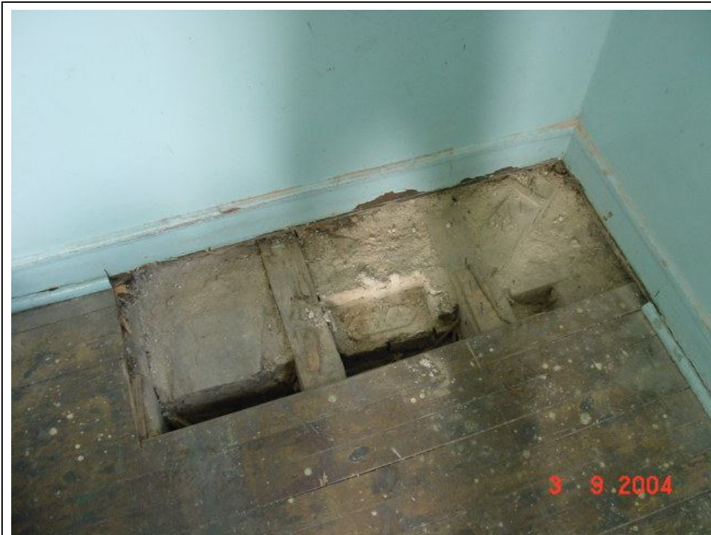
Description: Ph.68- Section cut of the timber floor at SE corner of room 12 showing timber beams supported directly to the basement wall below.
