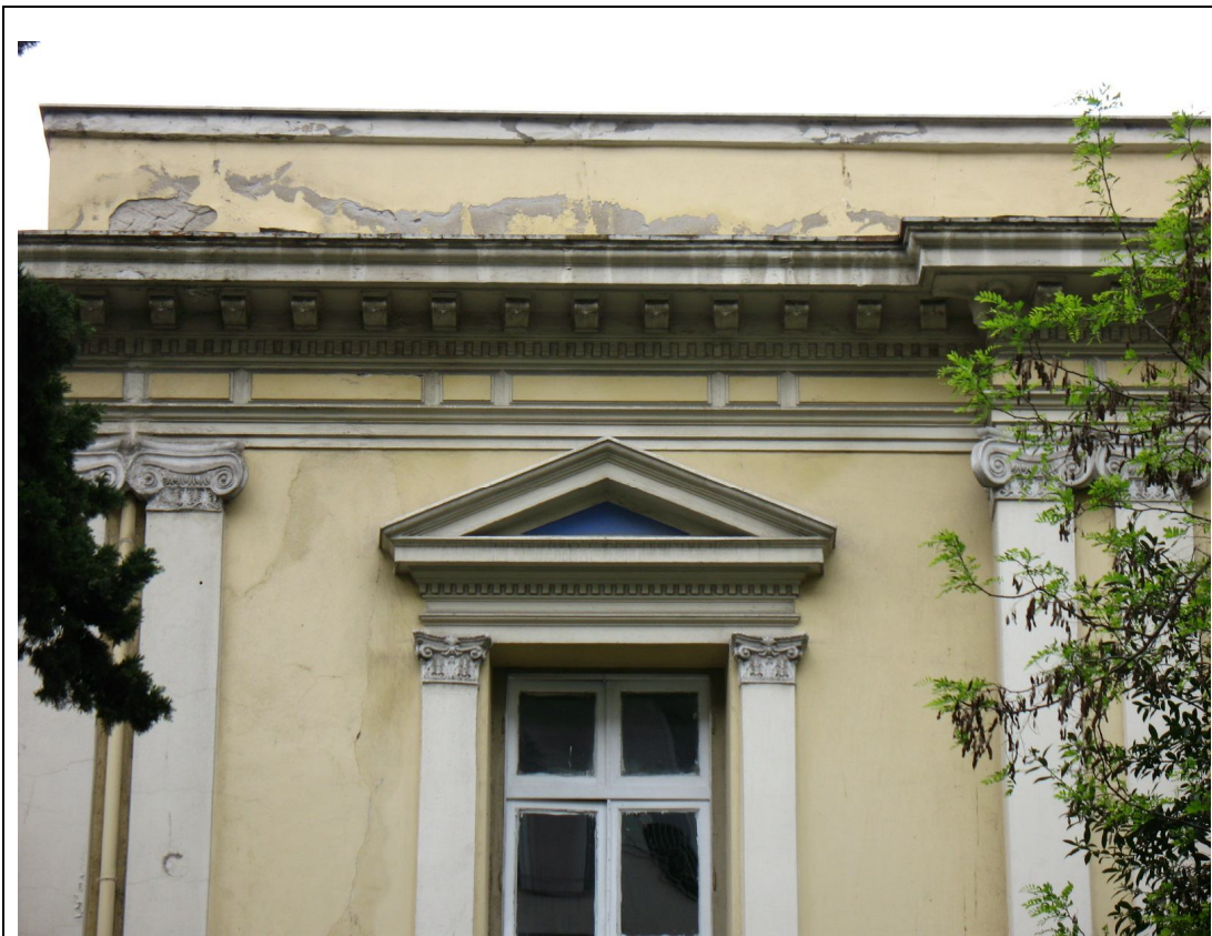
Description: Ph.4 – Detail of Photo 3 showing the disintegration of plaster along the parapet due to weathering conditions.
