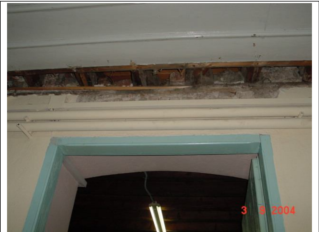
Description: Ph.71 - Section cut at the ceiling of room Y1 above the door entrance to room Y6. The timber ground floor beams are supported on a tie beam at the basement wall head.
