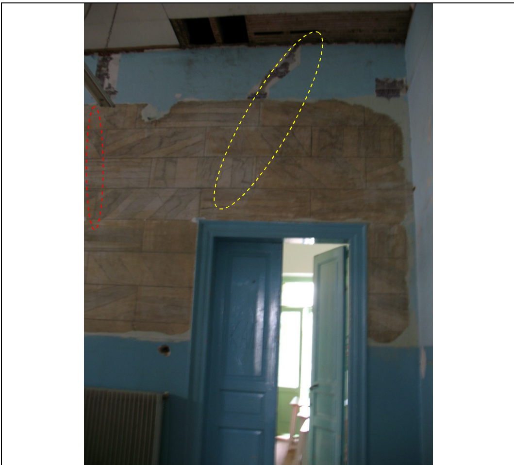
Description: Ph.23b- The right hand side of the wall from ph.23a showing the door entrance at room O6 and the cracks above door opening.
