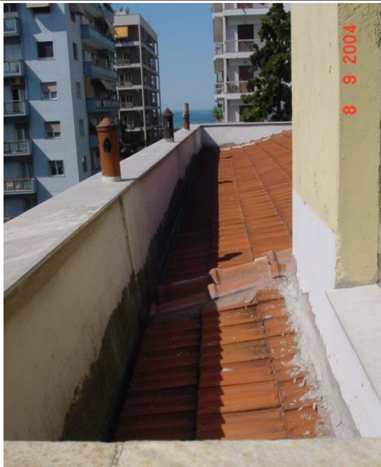
Description: Ph.43– Parapet inside view with the enclosed roof along the east elevation of the building. At the right hand side is shown the window of the staircase leading to the roof terrace.
