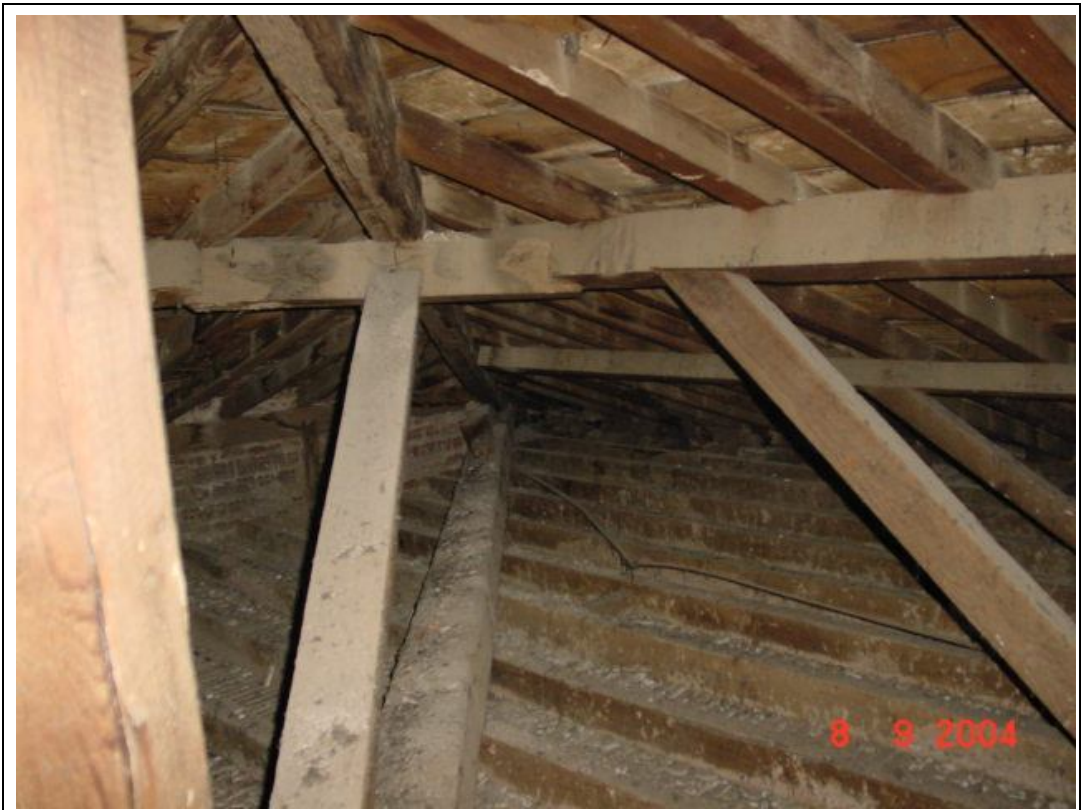
Description: Ph.48- NE view of the roof area inside showing the south wall of the staircase that leads to the roof terrace.
