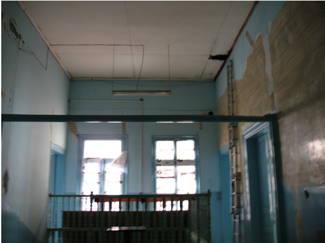
Description: Ph.20- Inside view of photo 18 – room O1 at 1 st floor level with the floor opening of the staircase.
