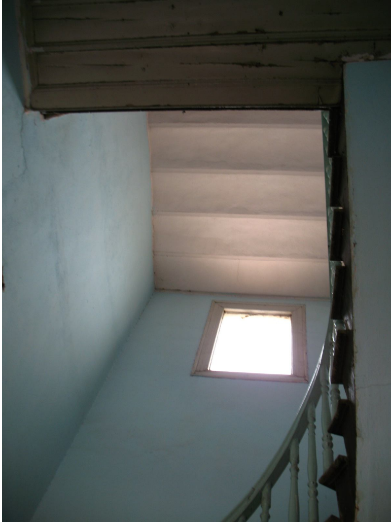
Description: Ph.28- Secondary timber staircase going to the terrace at roof level.
