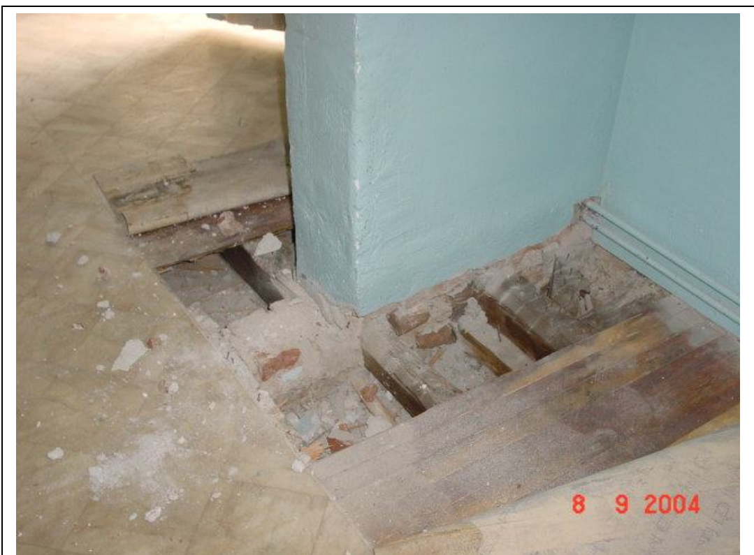
Description: Ph.60- Opened floor section at the bottom of the pier between rooms O1α – O2. It is shown the timber beams supported on the wall below between rooms I1-I2.
