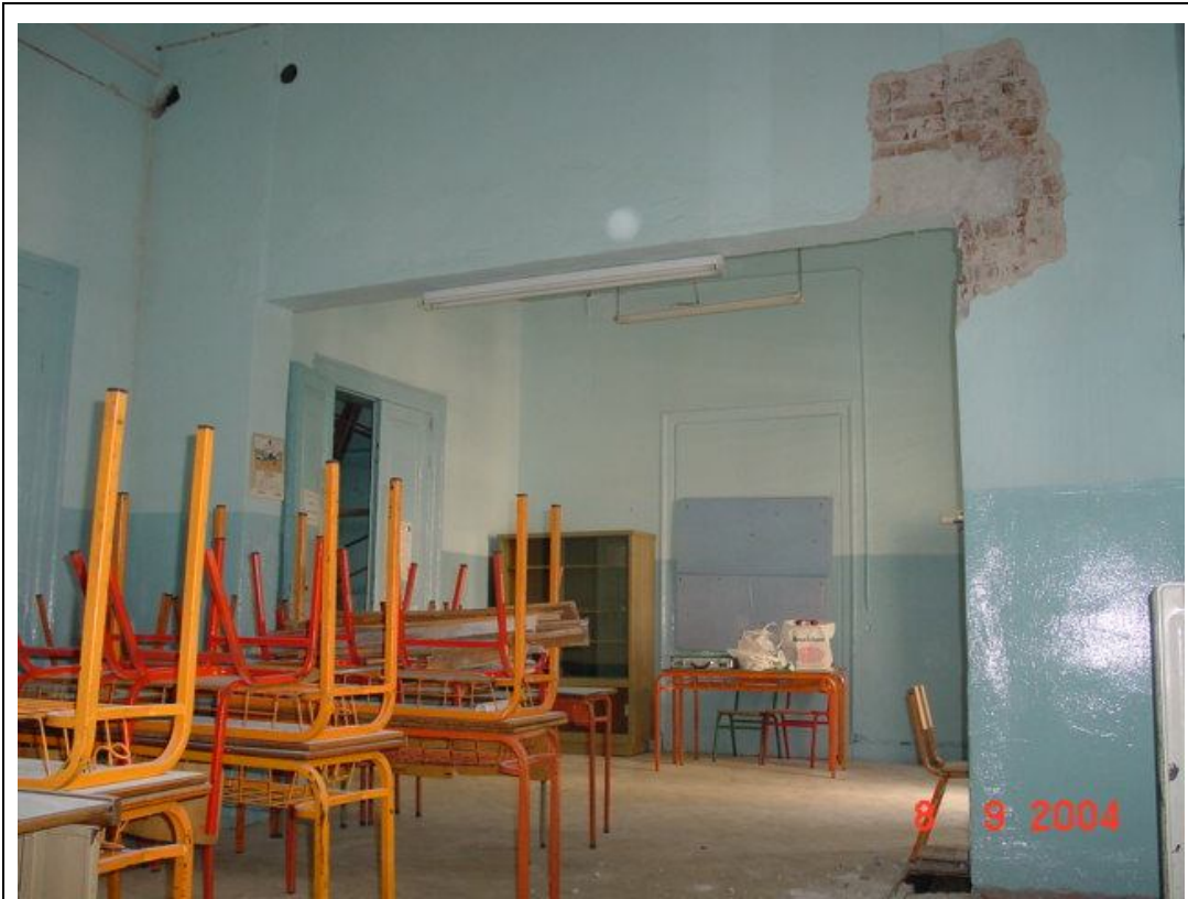
Description: Ph.59- View of the room O2 at 1 st floor showing the partial demolition of the wall between rooms O1α – O2.
