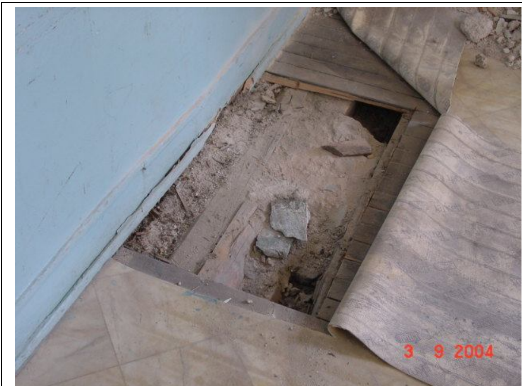
Description: Ph.69- Section cut of the timber ground floor between rooms 16 –17. The timber beams are supported directly to the basement wall below.
