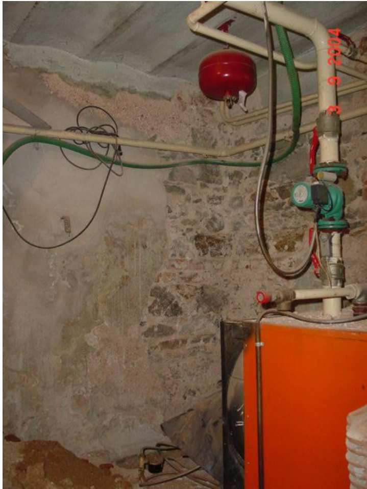
Description: Ph.74 – North side view of room Y10 at basement showing the rubble stone masonry and the arched floor between steel beams.
