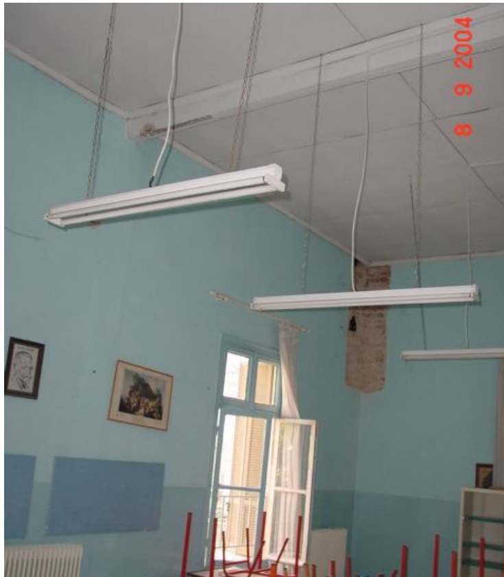
Description: Ph.57- View of the joined rooms O3 – O4 with the pair of steel beams at ceiling level to support the roof after the wall demolition.
