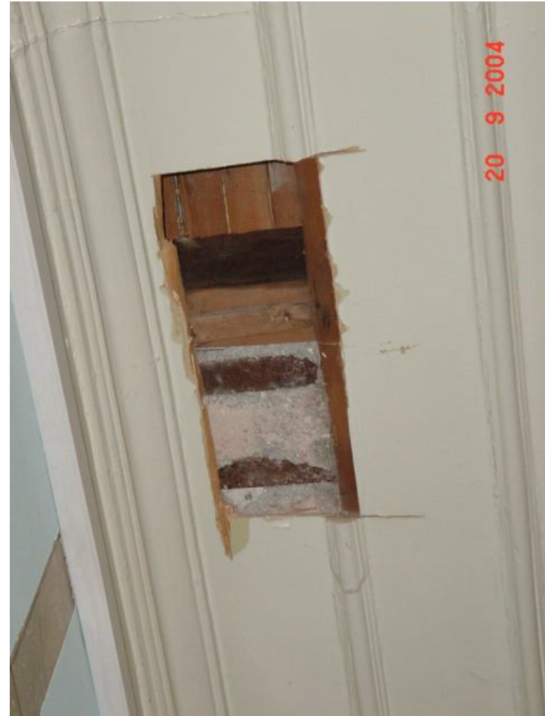
Description: Ph.61a- Detail of Ph.61 revealing the pair of steel beams that carries the wall above with the concrete infill between.
