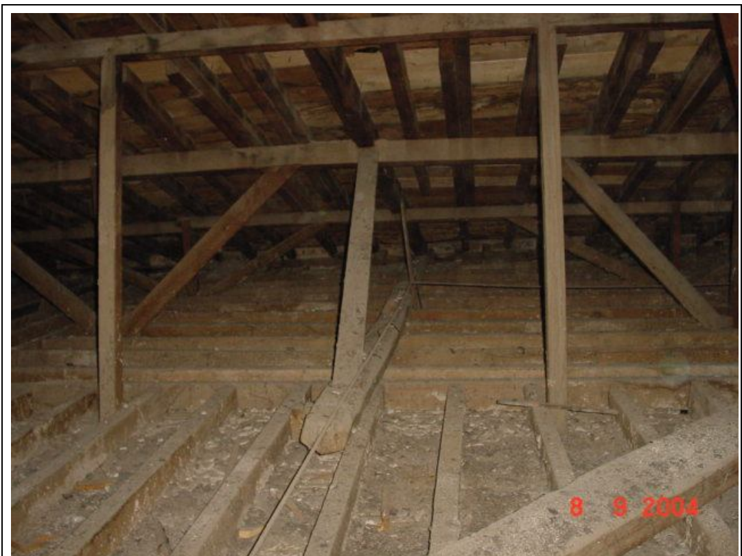
Description: Ph.49- View of the east area of the roof showing the secondary truss for the support of sloped roof elements.
