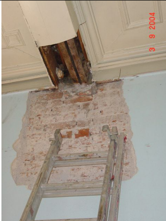
Description: Ph.66- Detail of Ph.65 showing the surface corrosion of the double steel beams I140 that support the timber beam above which then act as a line of support for the timber floor beams at room O6-O7.
