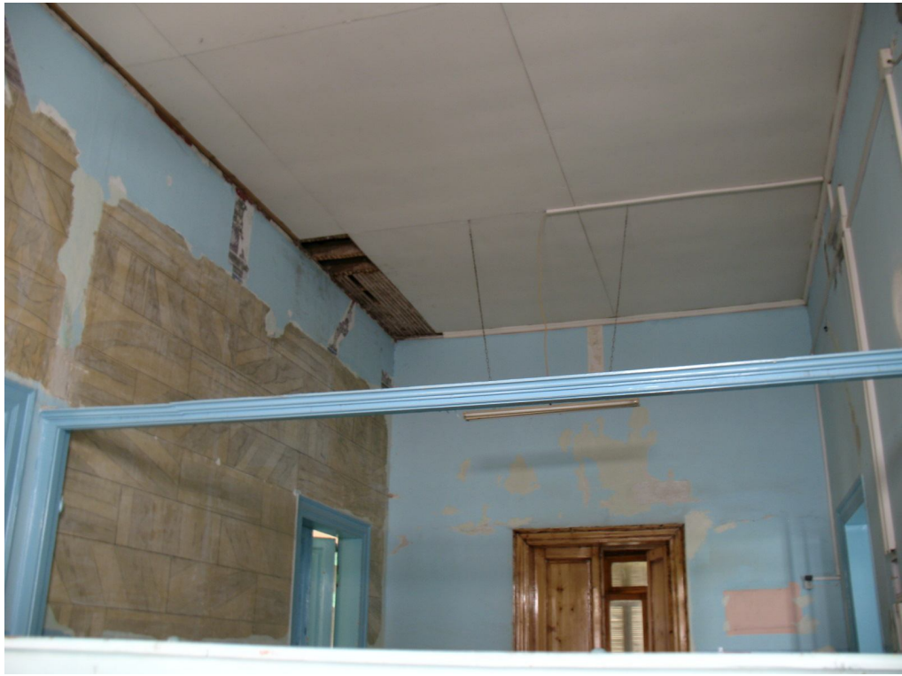
Description: Ph.22- Opposite view (from ph.20) at room O1 from the corridor O11 showing the door entrances at rooms O1 \alpha and O6 (left).
