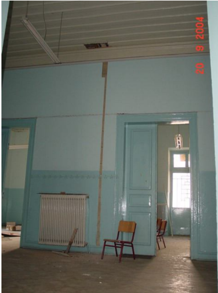
Description: Ph.61- Location of the ground ceiling at room I1 (under the 1st floor wall between rooms O1 – O1α).
