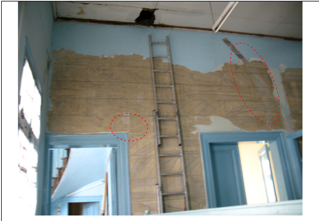
Description: Ph.23a- Front view of the wall of ph.23 (room O1) with cracks above openings.
