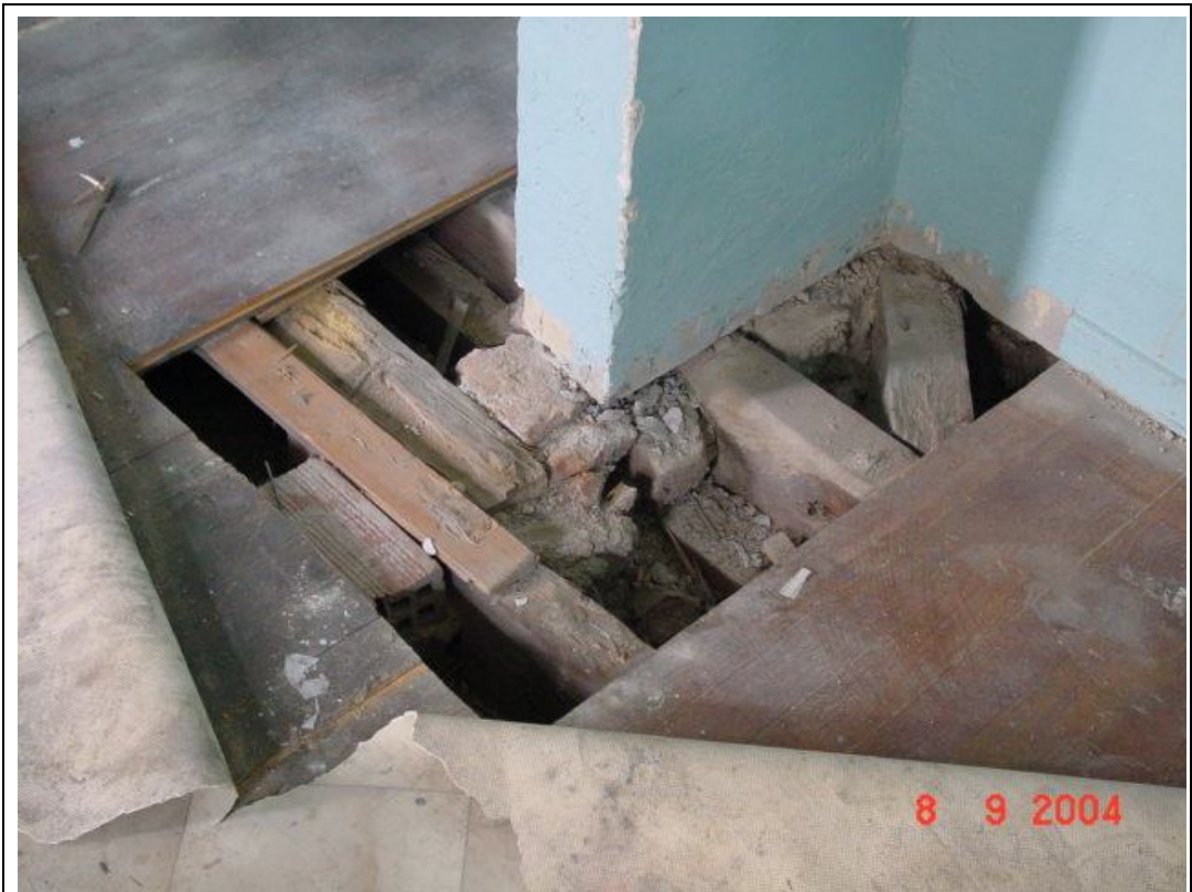
Description: Ph.54- Exposed floor section between rooms O5 – O6 showing the transverse timber beams being supported directly to the ground floor wall.
