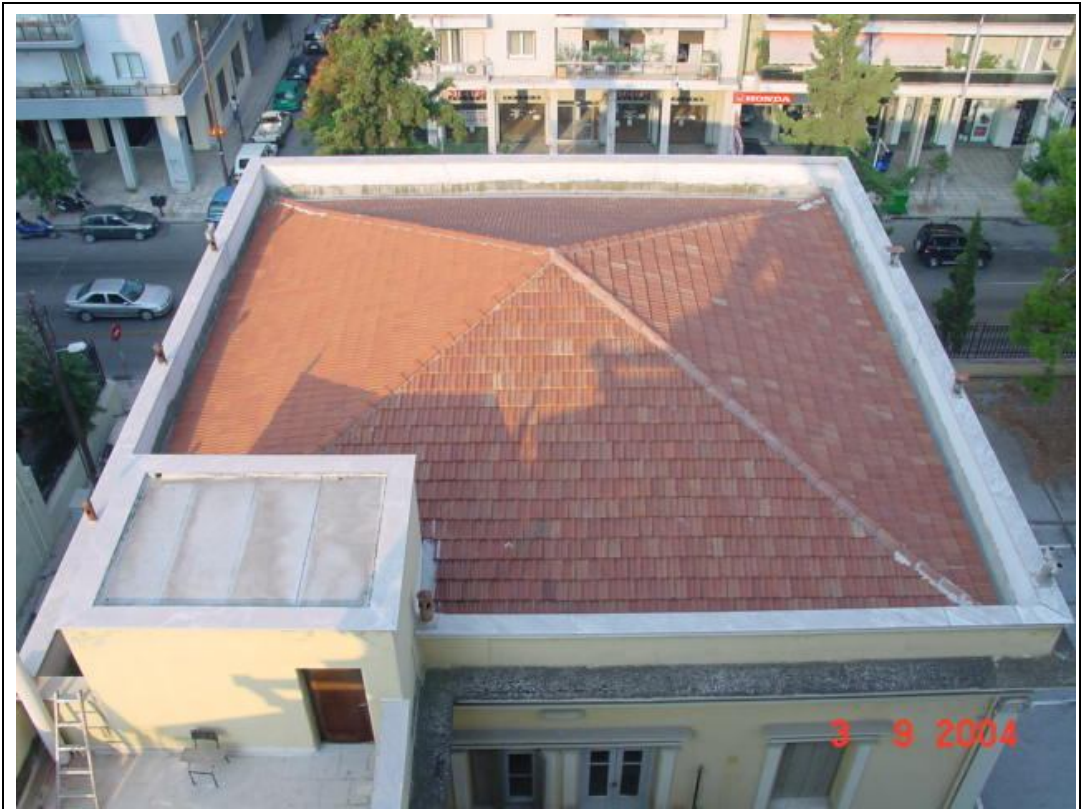
Description: Ph.42– Panoramic view of the hipped roof and terrace of the building.
