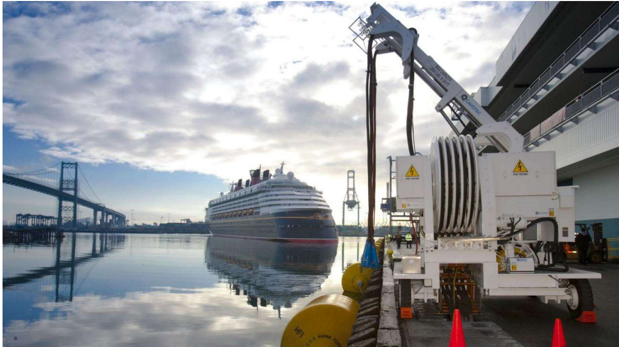
Shore power at the Port of Los Angeles
