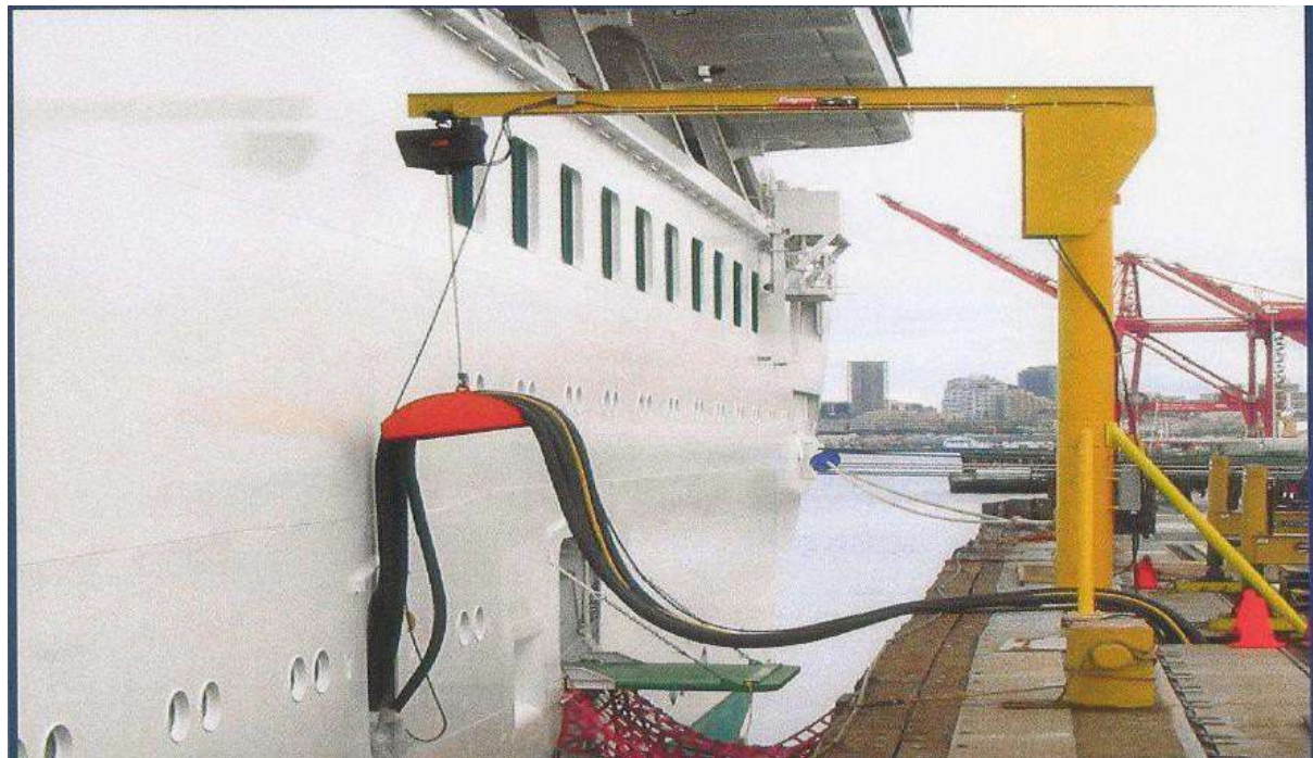
Power Cables at the Port of Seattle
