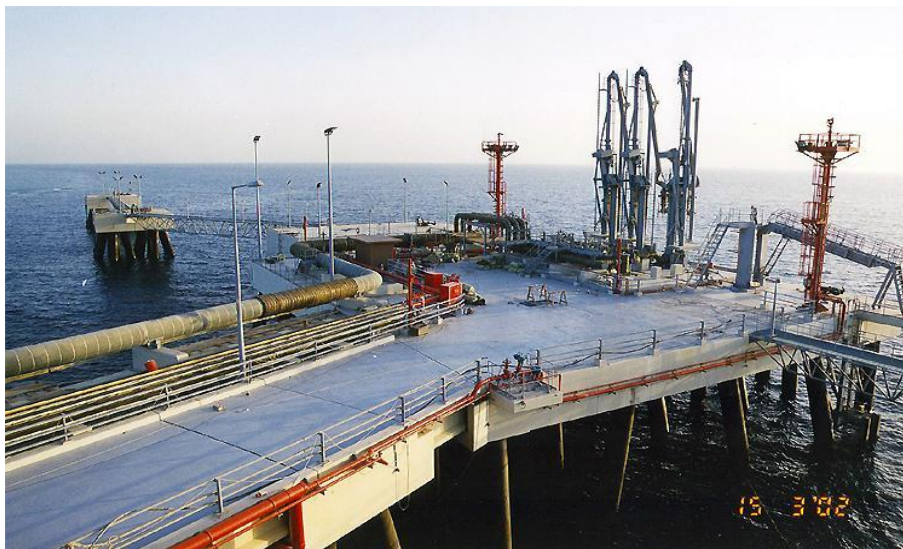
iii. Tanker terminal- Shoaiba Desal Plant
