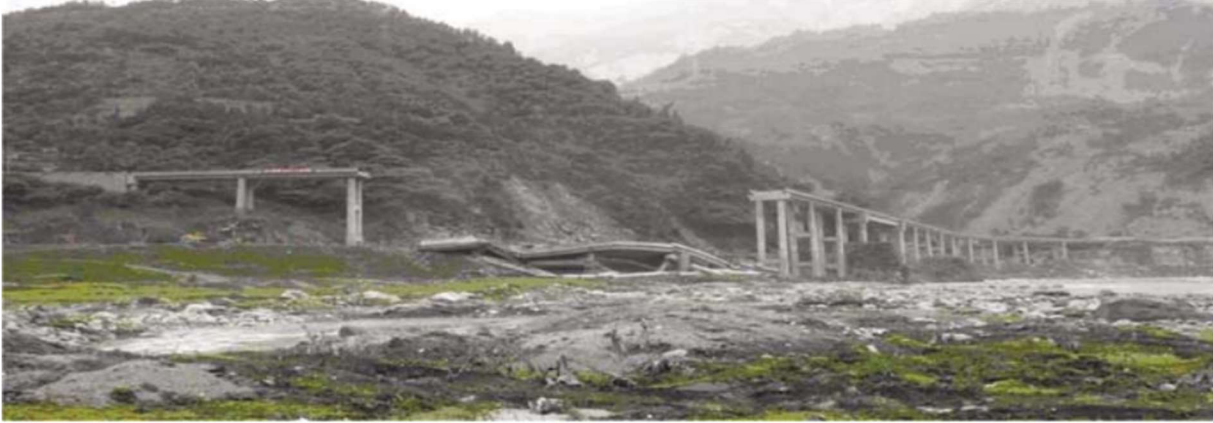
Figure 22 Failure of the Baihua Bridg
